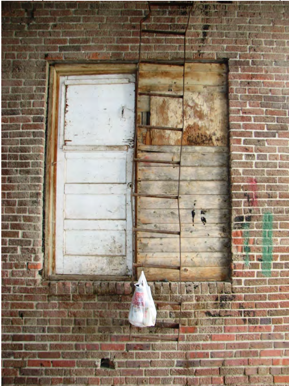
Photo MT_FergusCounty_Gamble-RobinsonCoWarehouse_0005. North "Rear" Elevation, Detail of Elevated Truck Loading Dock, facing: SE
