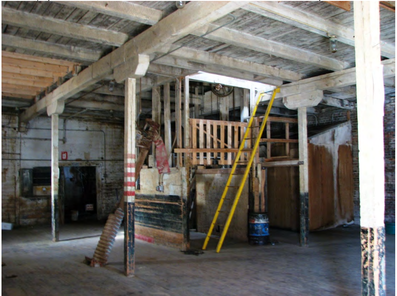
Photo MT_FergusCounty_Gamble-RobinsonCoWarehouse_0009. Interior, Main Floor Warehouse Space with Freight Elevator, facing: N
