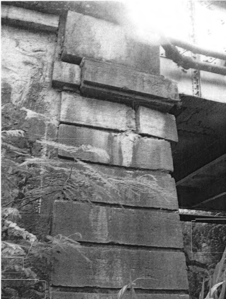
Close up photo of the bridge's abutment taken by José E. Marull, PRSHPO, September 18, 2008.
