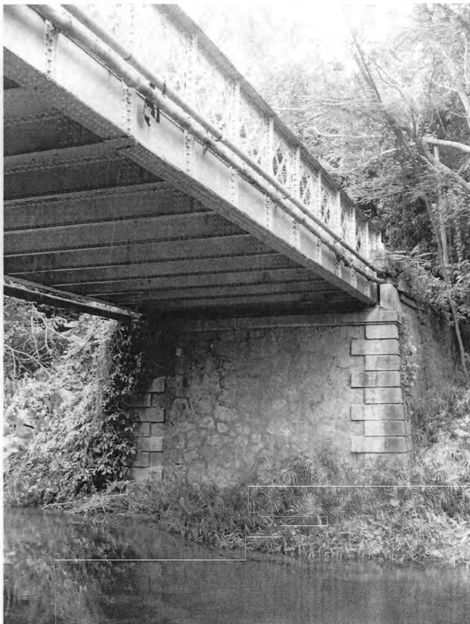
Photo of the deck and abutment of the bridge over the Cuyón River. Taken by José E. Marull, PRSHPO, September 18, 2008.
