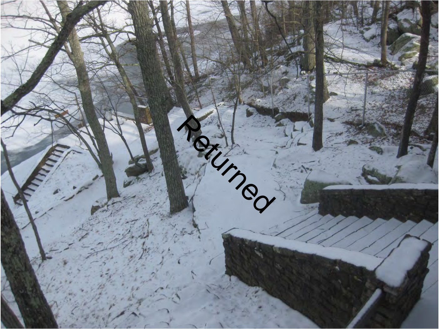
Photo 9: Stonework, terracing and steps between the bathhouse and the lake, camera facing north
