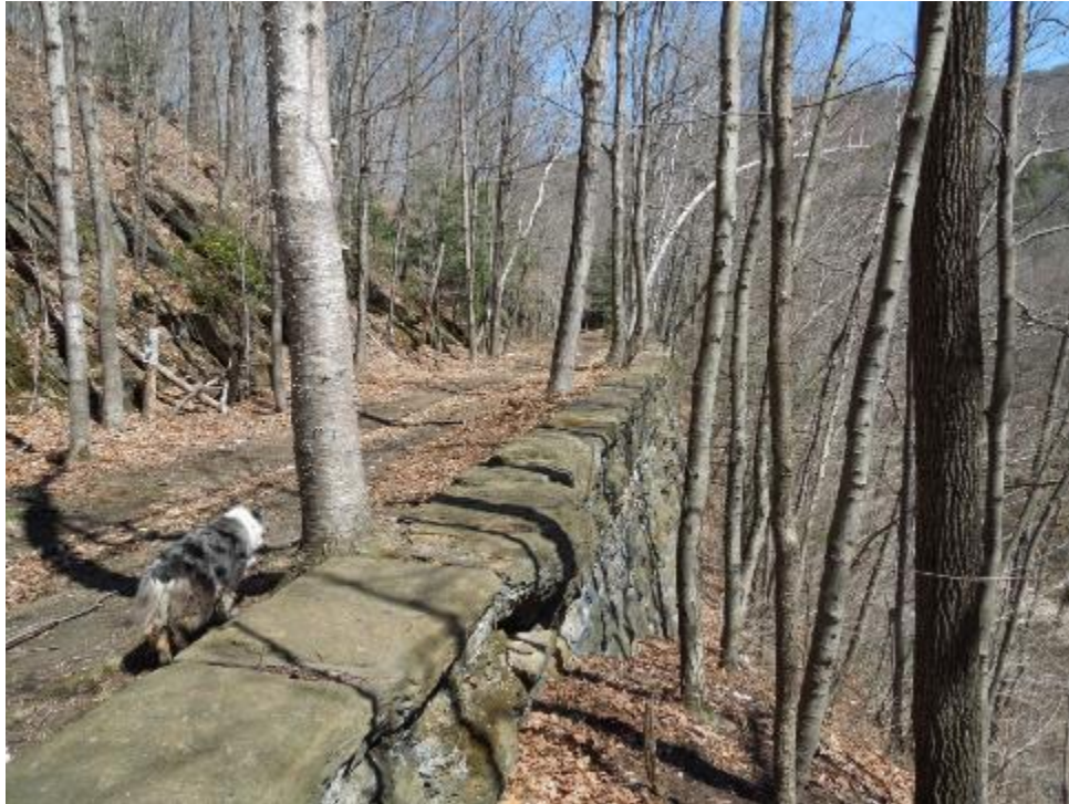
9. Embankment and retaining wall of Western Railroad Roadbed between Bridges No. 5 and 6, looking east. Roger Reed, NPS, 2014.
