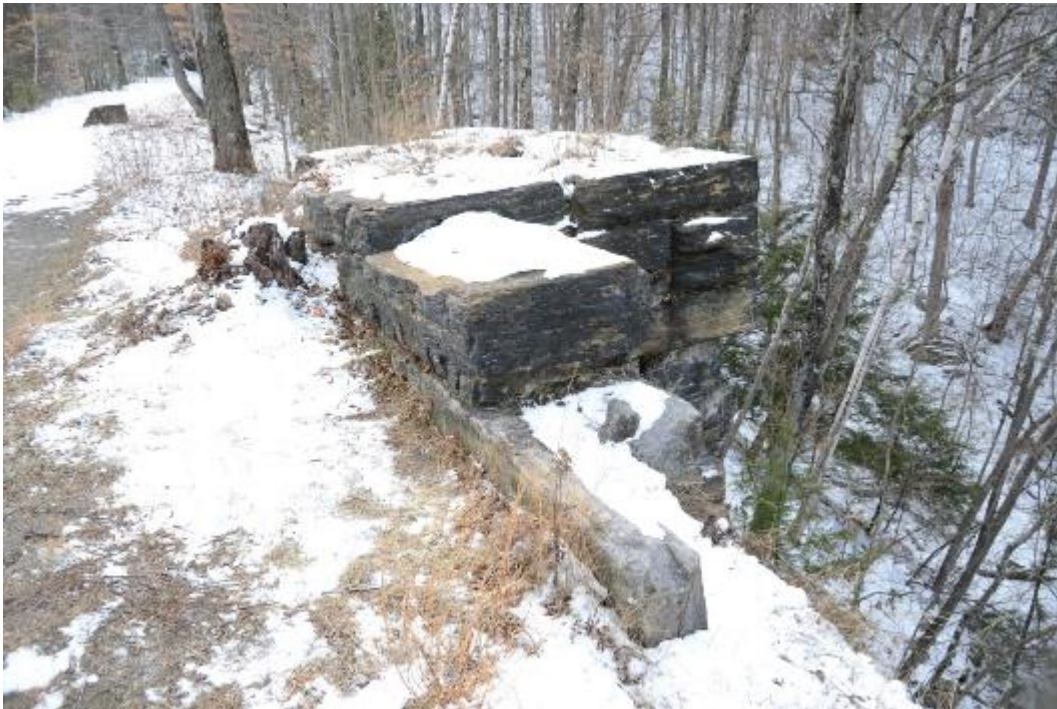
14. Detail of northwest pier and parapet remnant on Bridge No. 5, looking northwest. John Daly, PAL, 2017.
