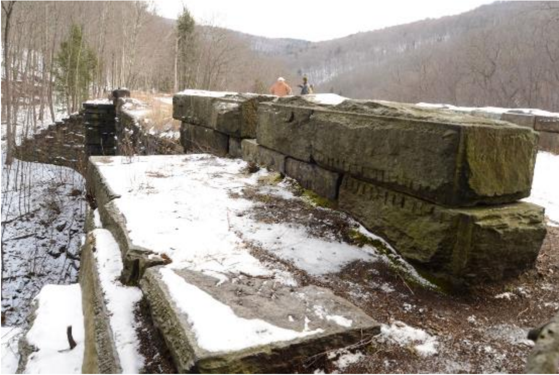
7. North parapet and date stone of Bridge No. 6, looking southeast. John Daly, PAL, 2017.
