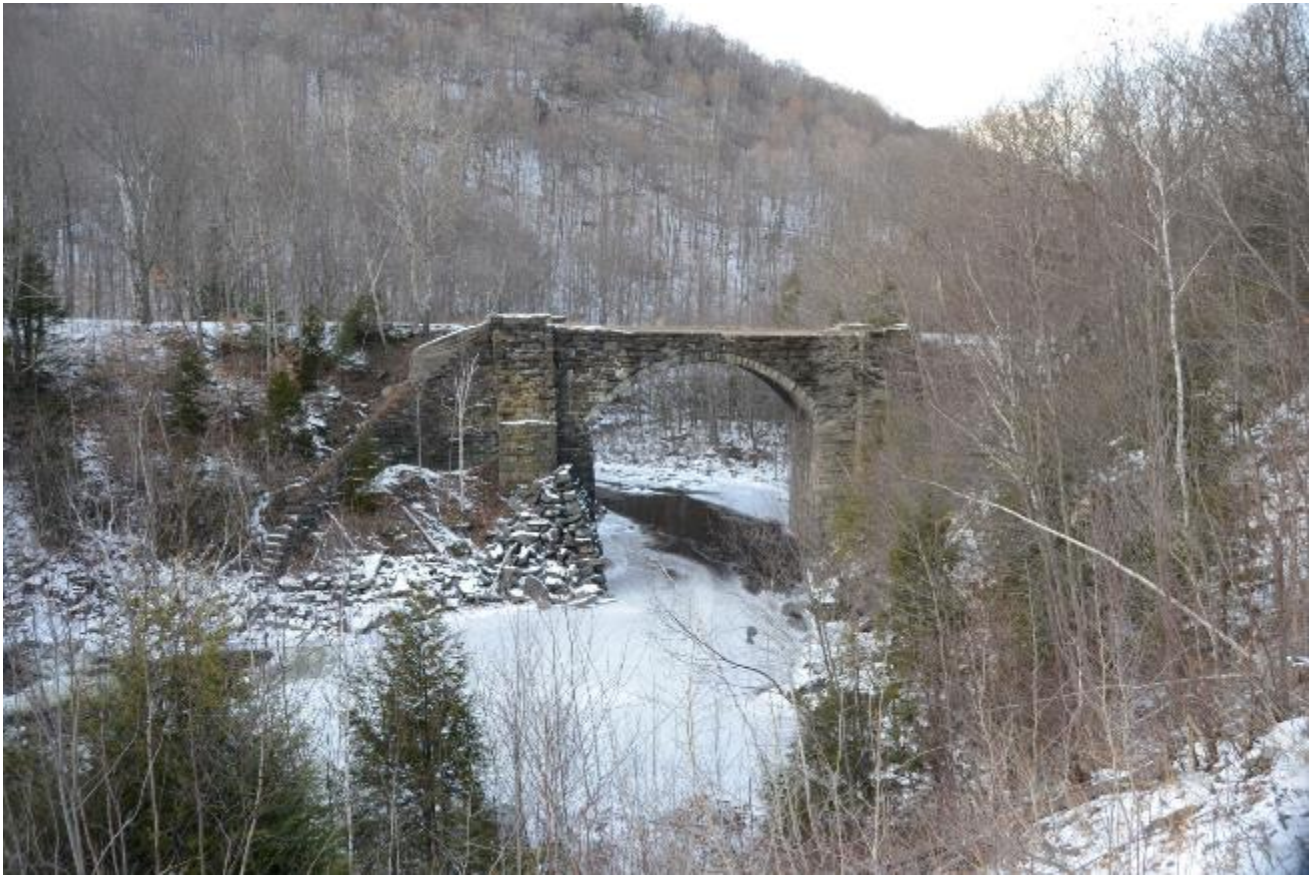
10. Western Railroad Roadbed and Western Railroad Stone Arch Bridge No. 5 (Bridge No. 5) in the Westfield River gorge, looking north (downstream). John Daly, PAL 2017.
