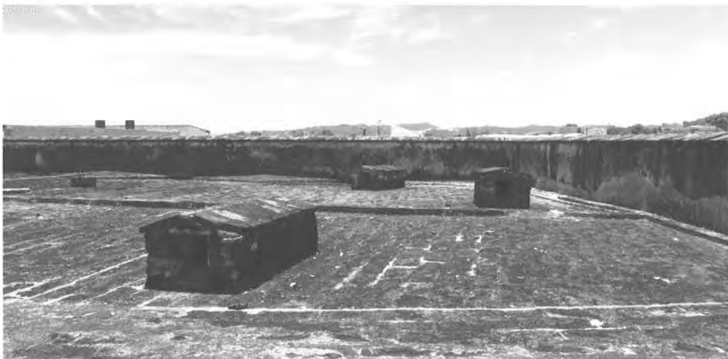
Fig. 9 Ventilation structures at the roof.
