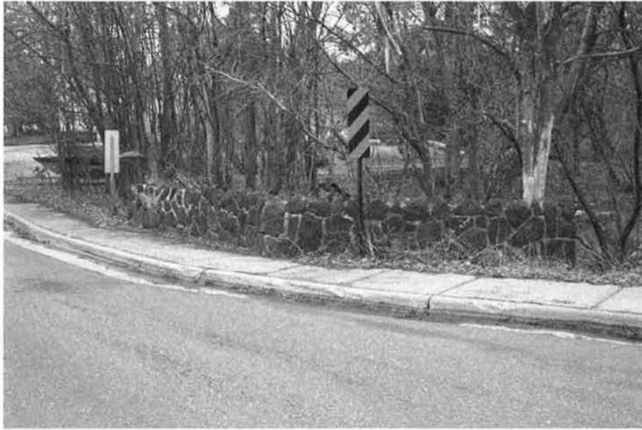
Photo 5 of 10 MN_St. Louis County_Bridge No. L8515_0005 Bridge No. L8515, north railing. Facing northwest.
