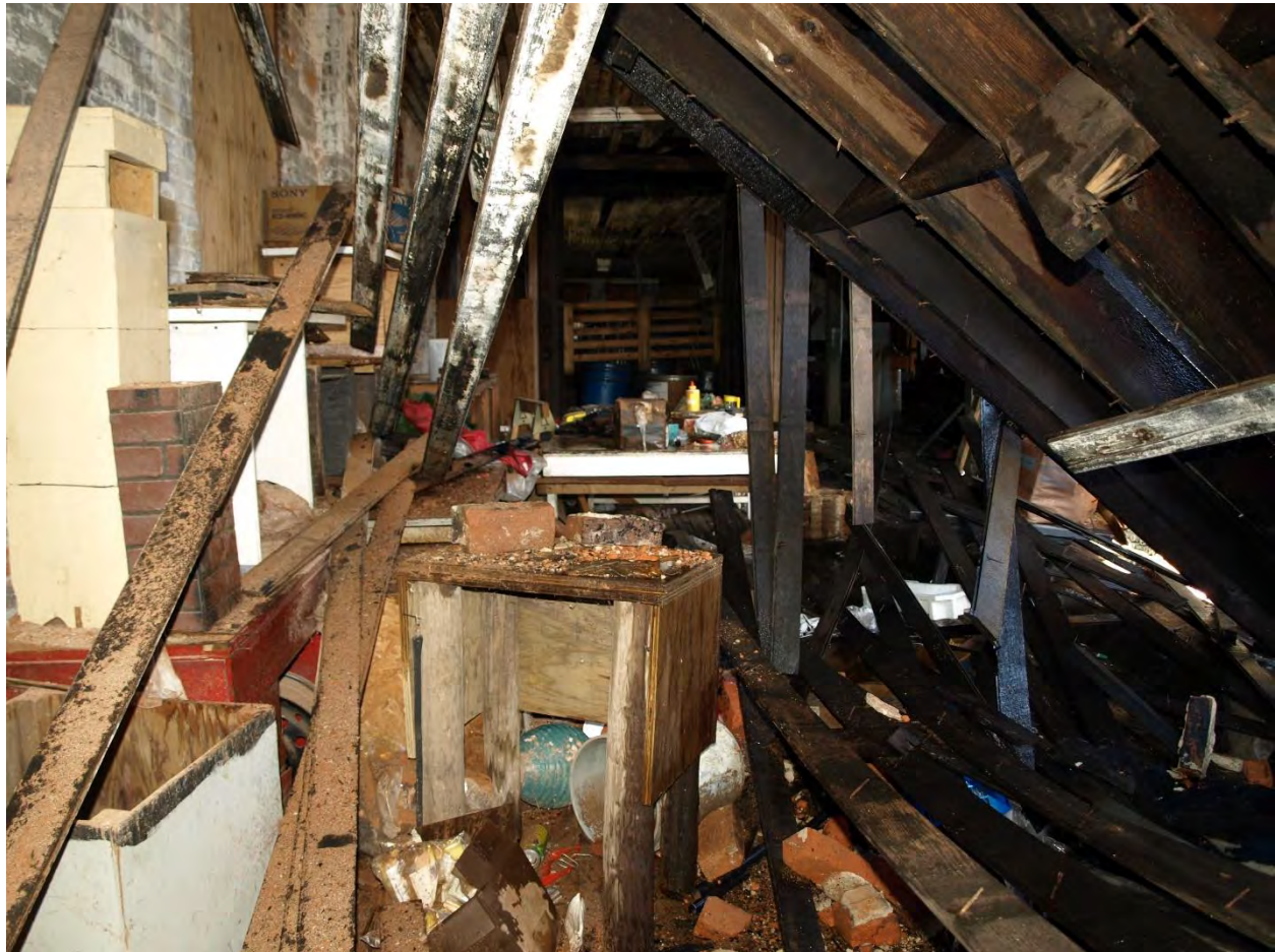
Fig. 15: Second floor after second roof collapse, looking southwest toward front of building. (Source: Laura Sadowsky, site visit, August 5, 2016.)
