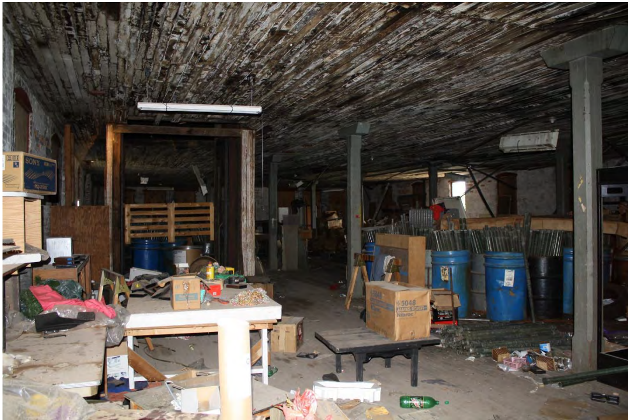
Fig. 13: Photo of second floor prior to roof collapse. (Source: Mary Ottoson, Hobart Historic Restoration, August 8, 2014.)
