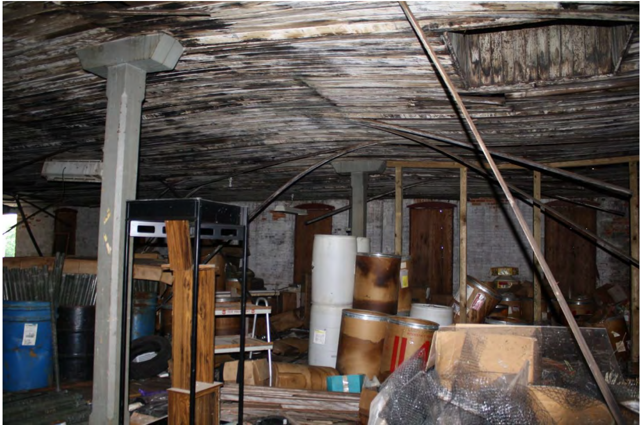
Fig. 14: Photo of second floor prior to roof collapse. Note chamfered, heavy timber support posts. (Source: Mary Ottoson, Hobart Historic Restoration, August 8, 2014.)
