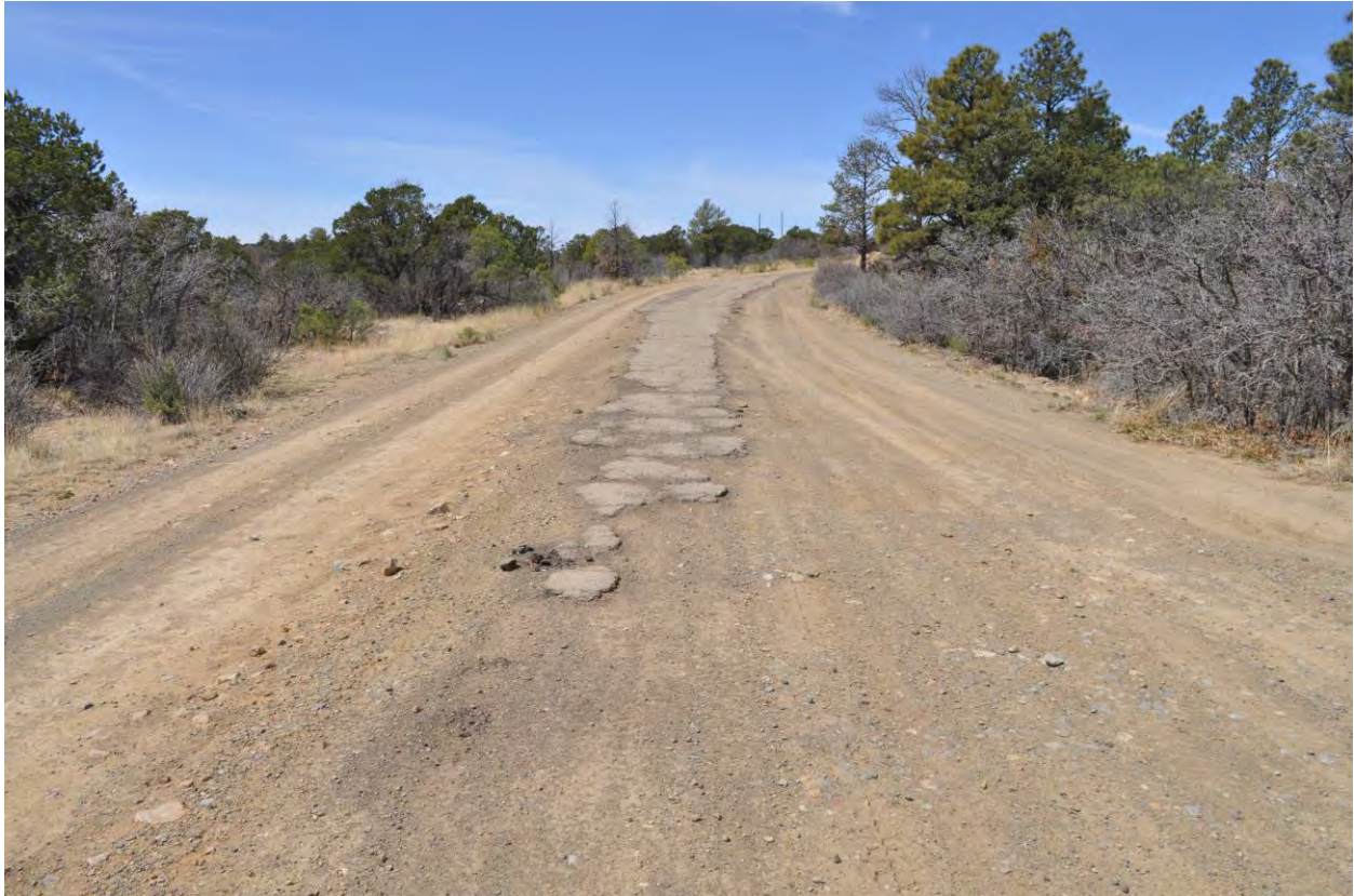
16 of 16: Beyond historic district boundary, deteriorated road conditions, photographer facing northwest.
