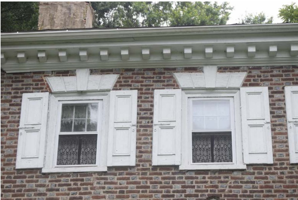
Photo 8. Close-up of second story windows of original block showing paneled shutters and flat-arched wood lintels with keystone toward northwest.
