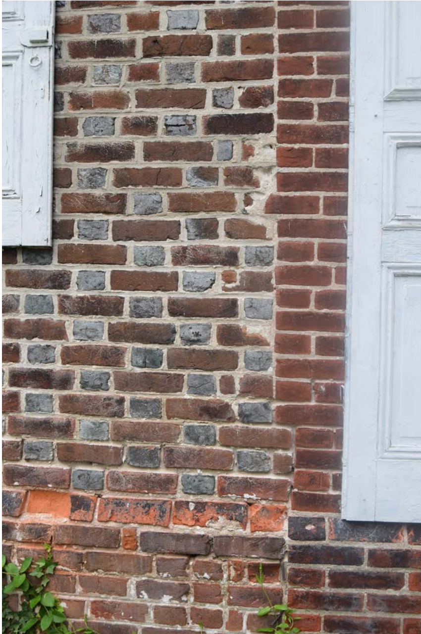
Photo 5. Close-up of brickwork of original block showing Flemish bond and water table toward northwest.
