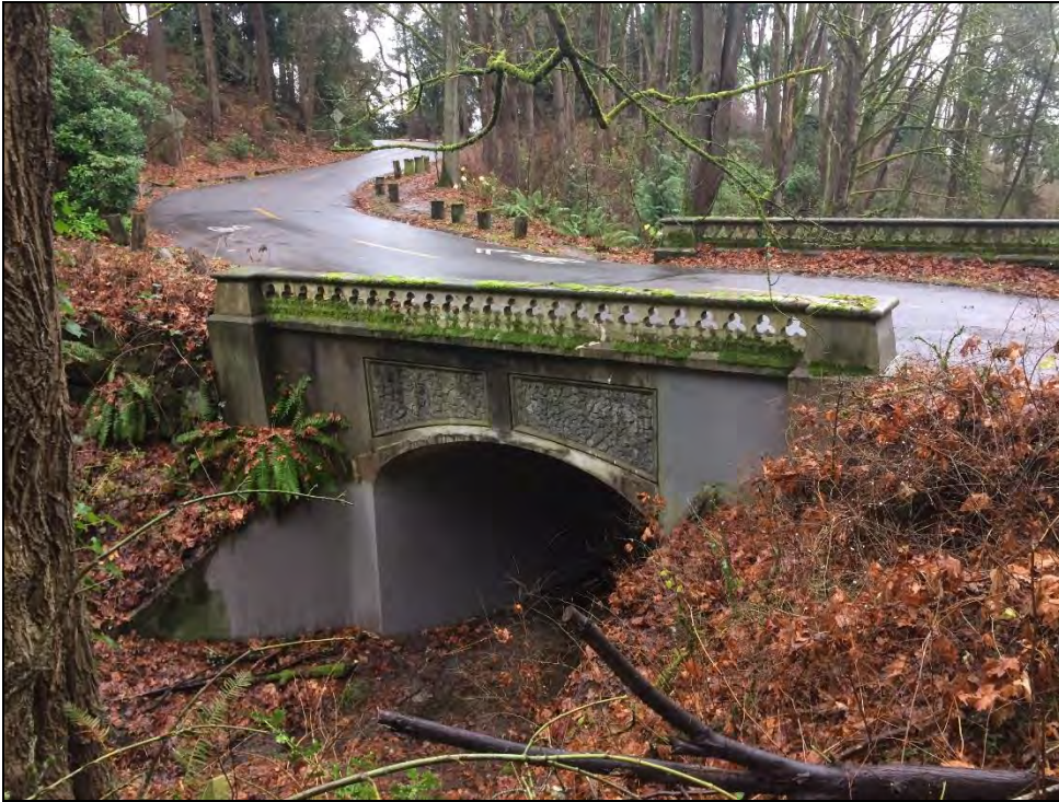
No. 0008, looking northeast at the concrete bridge and Lake Washington Boulevard S (December 18, 2017).
