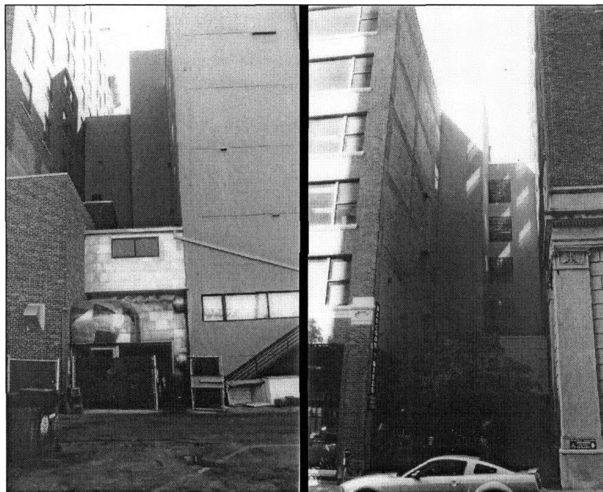
Figure 11: Connecting infill on north side, view east from alley (left), view west from 10 th Street (right) (photographs by James Jacobsen, March 2008)
