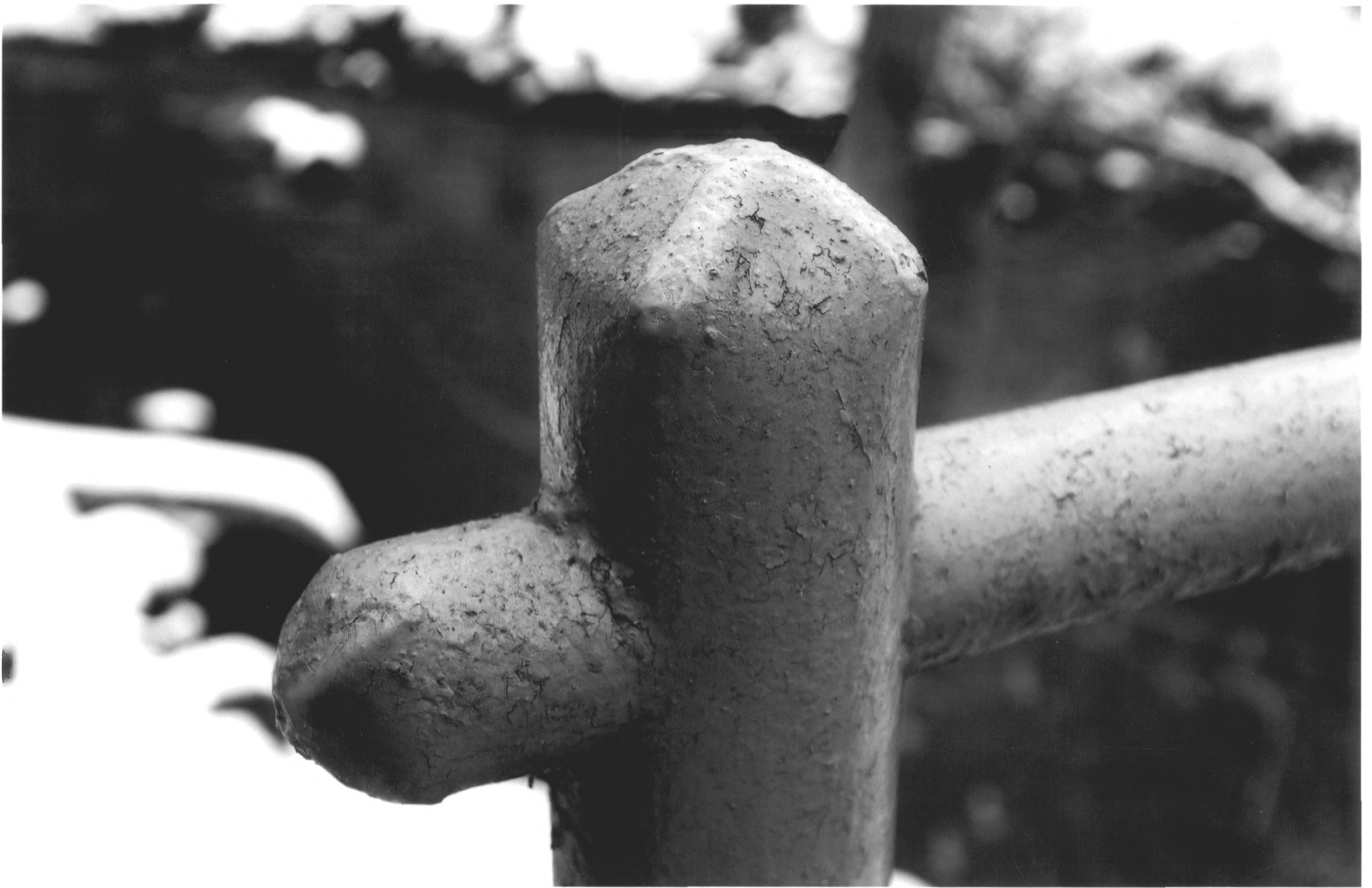
Perry Avenue Bridge Norwalk, Fairfield County, Connecticut Photograph 6 post detail December 11, 2005 Tod Bryant
