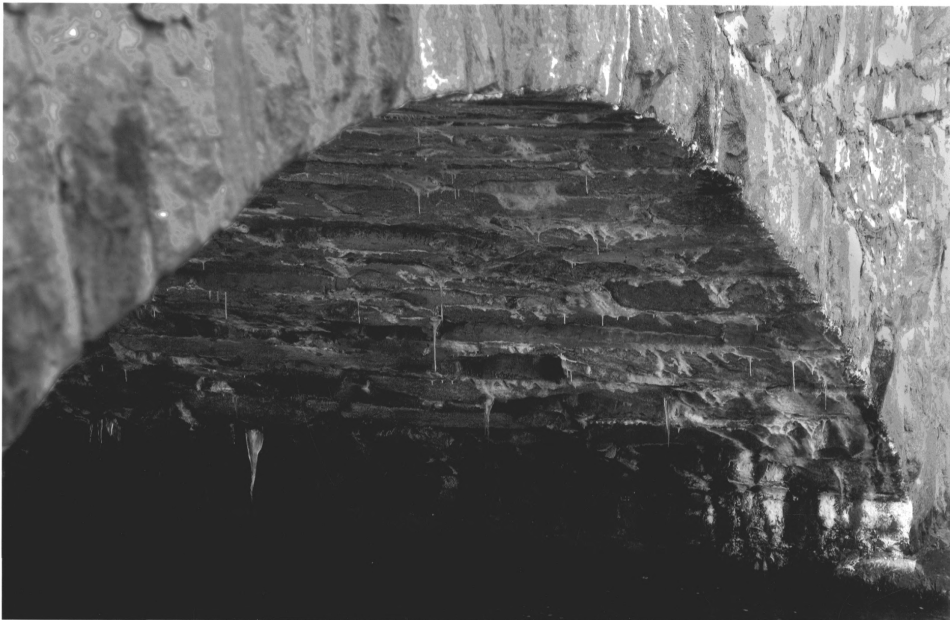
Perry Avenue Bridge Norwalk, Fairfield County, Connecticut Photograph 8 intrados December 11, 2005 Tod Bryant
