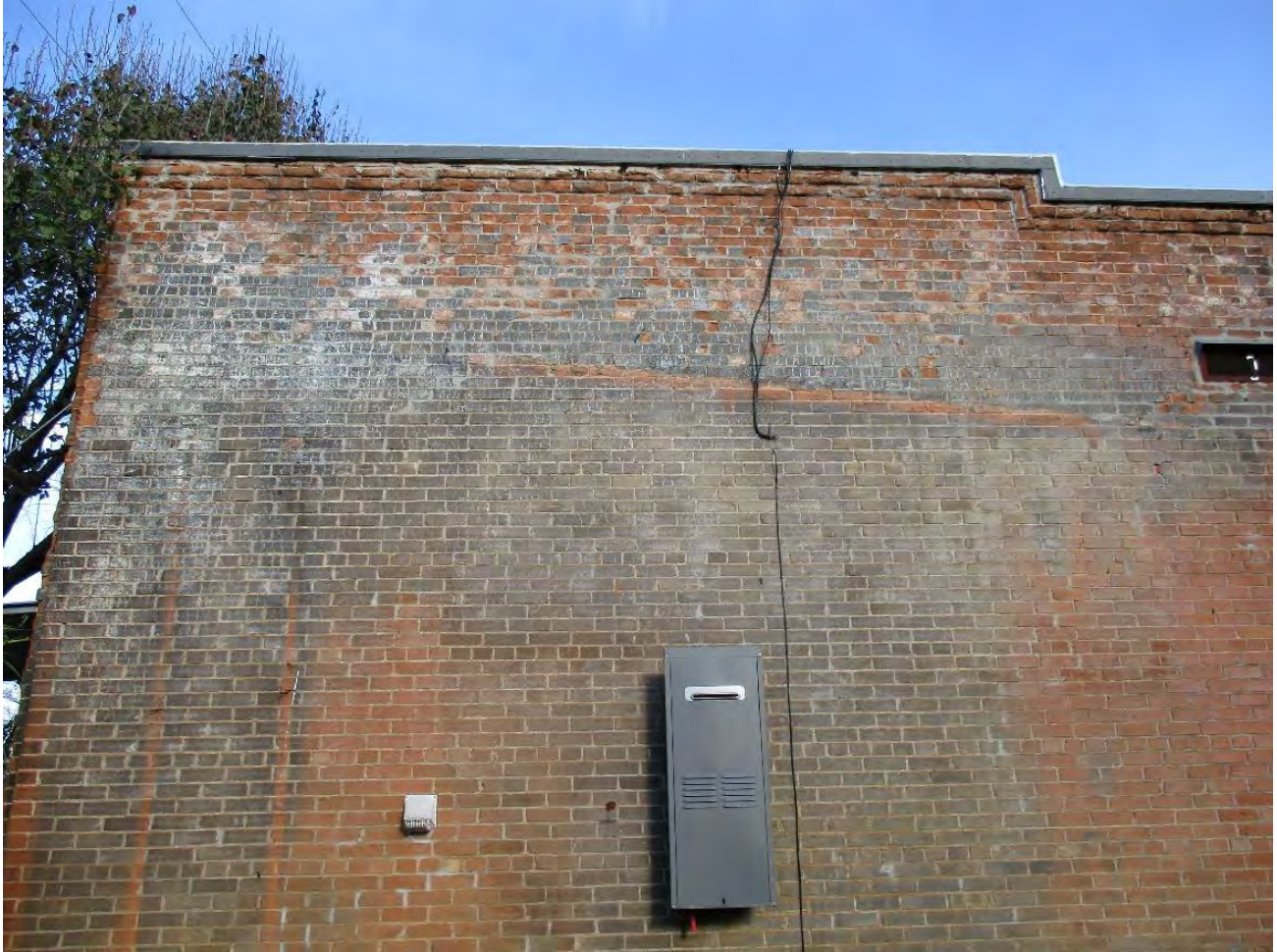
Photo 4: West elevation of Mangham-McIlwain Building showing fire damage. Camera facing east.
