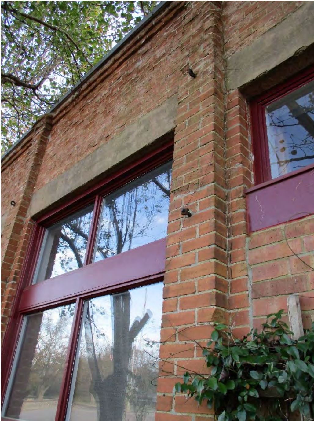
Photo 3: North façade of Mangham-McIlwain Building, detail of metal awning supports. Camera facing southeast.
