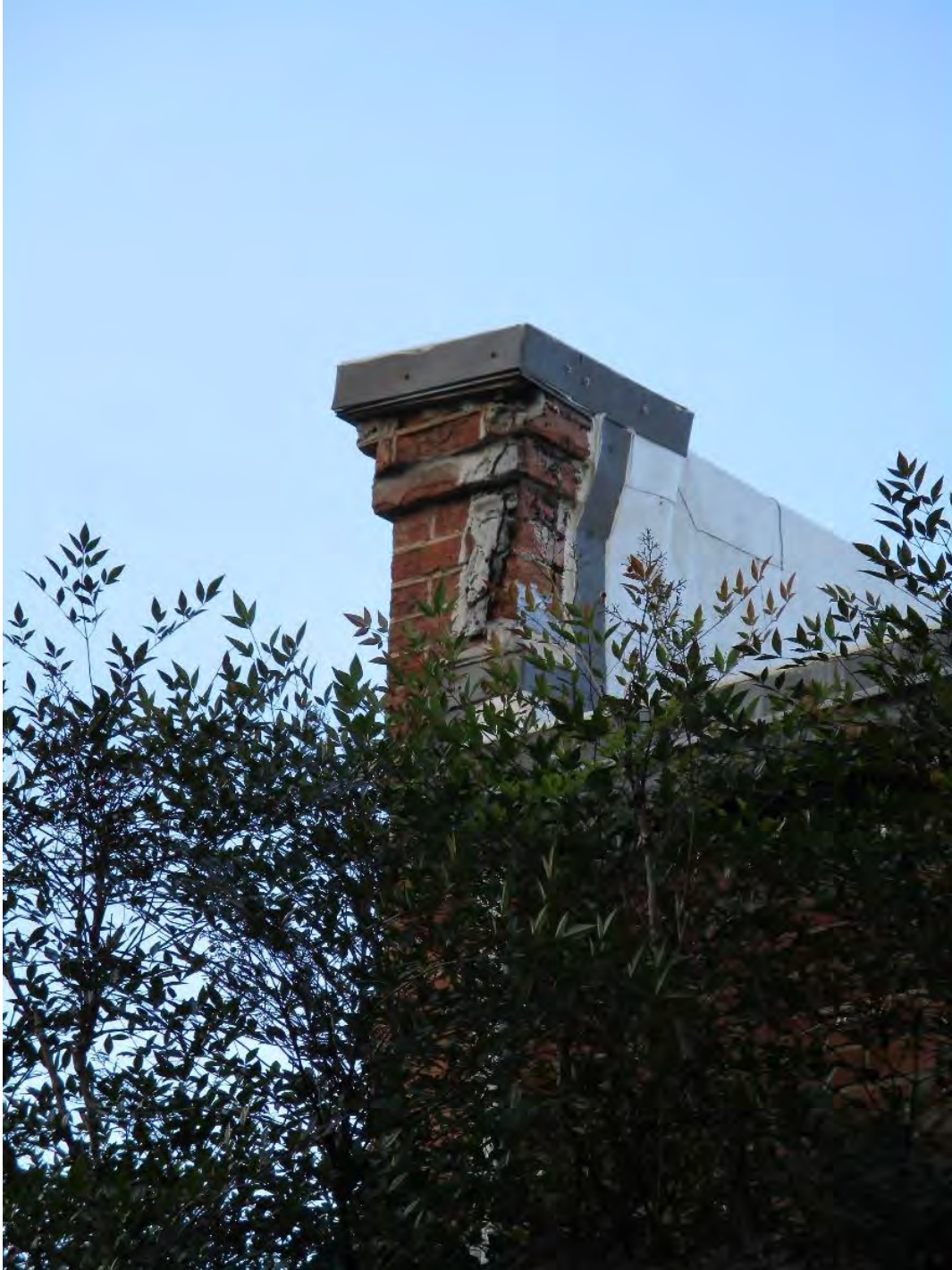
Photo 10: Top section of southern end of western elevation showing capped brick of Mangham-McIlwain Building. Camera facing northwest.
