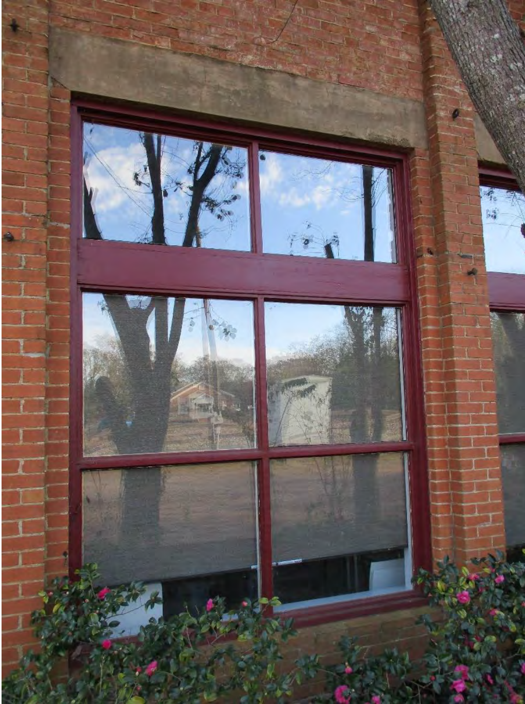
Photo 7: Detail of first window west of entrance on north façade of Mangham-McIlwain Building. Camera facing south.
