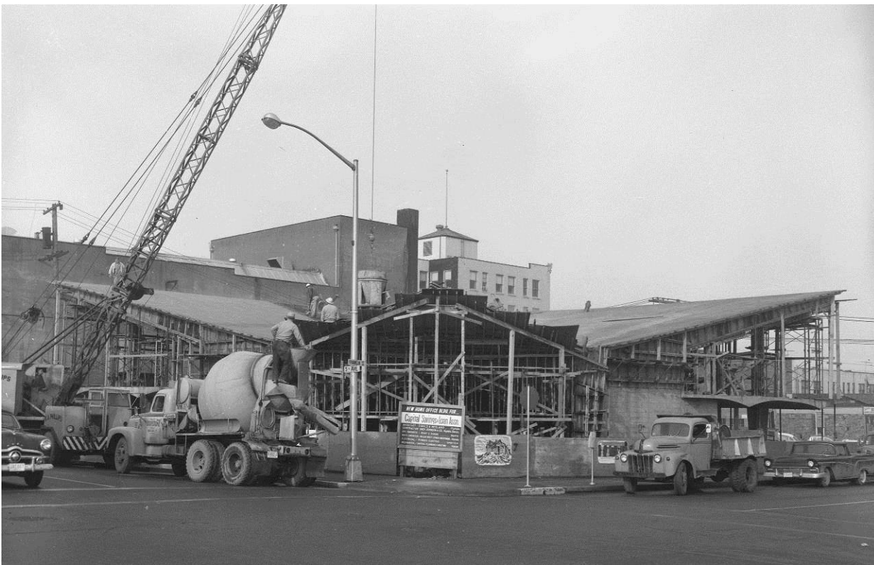
Capital Savings & Loan - construction photo – January 17, 1963 Images Courtesy of WA State Archives – Parish Collection
