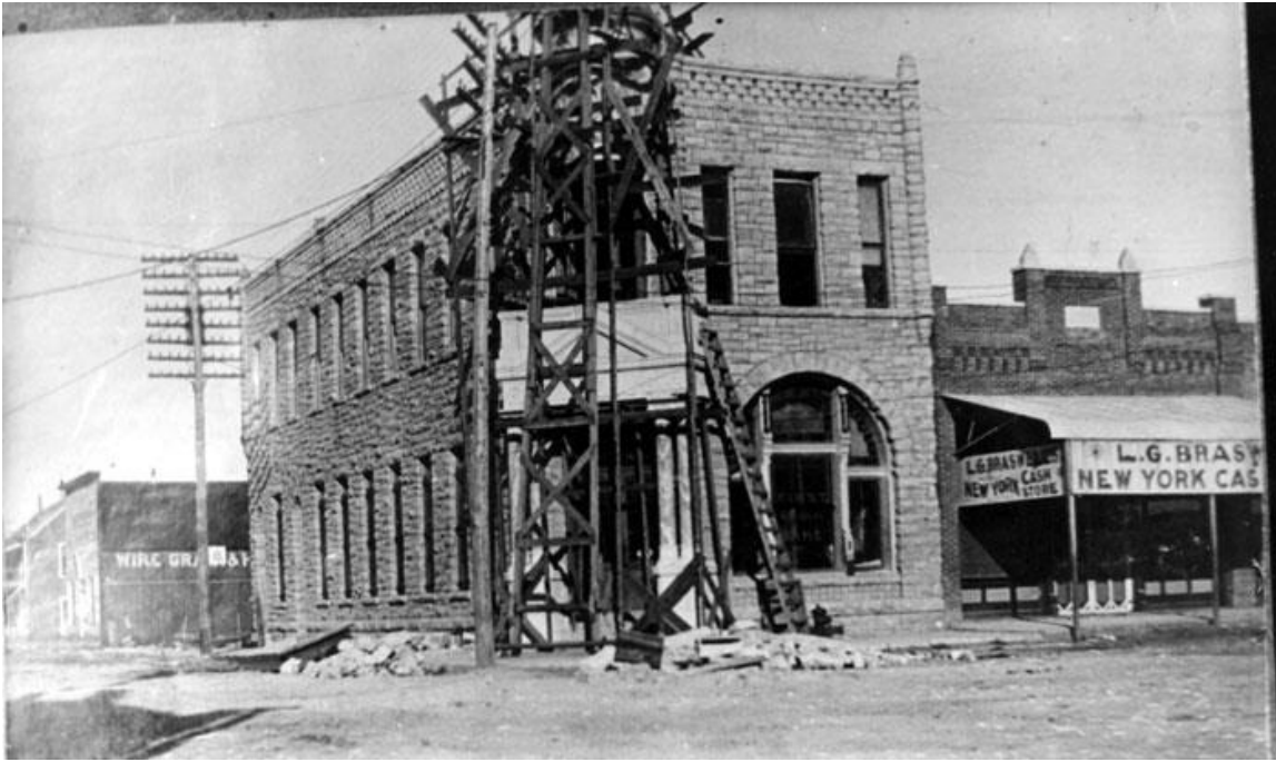
Figure 3 - Exterior view of First National Bank Building during reconstruction of corner, following fire; c. 1902. Camera facing northwest
