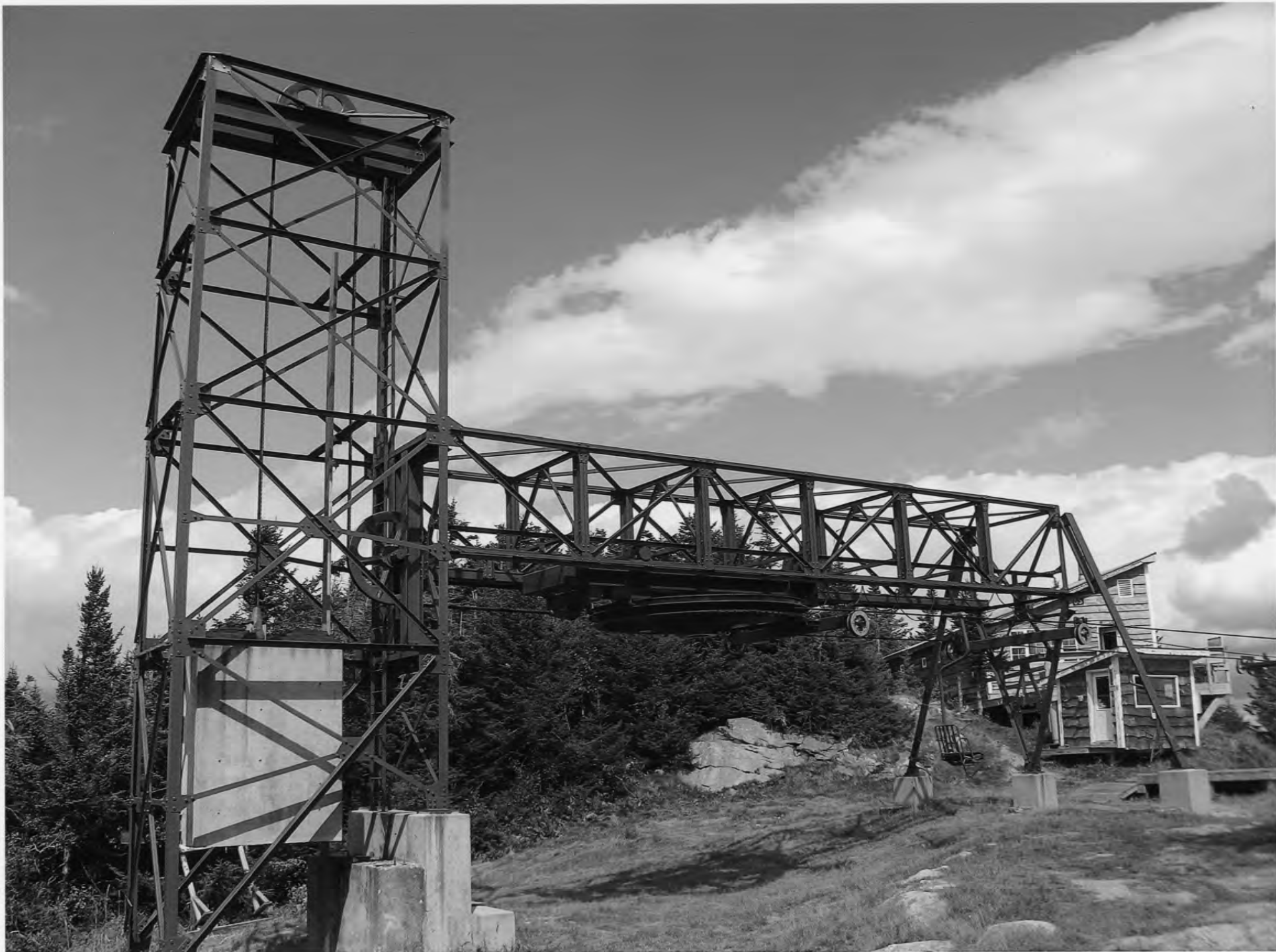
Mad River Glen Ski Area Historic District, Fayston, Washington Co. & Buel's Gore, Chittenden Co., Vermont
