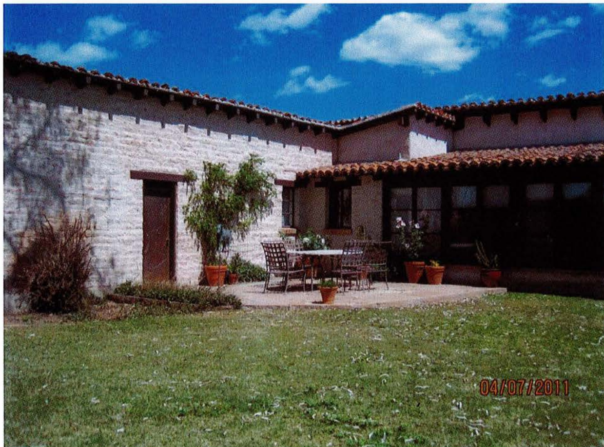
Photo #6 (AZ_PimaCounty_CFEJob#399House_0006) Rear (south) façade showing glass enclosed sunroom, camera facing north.
