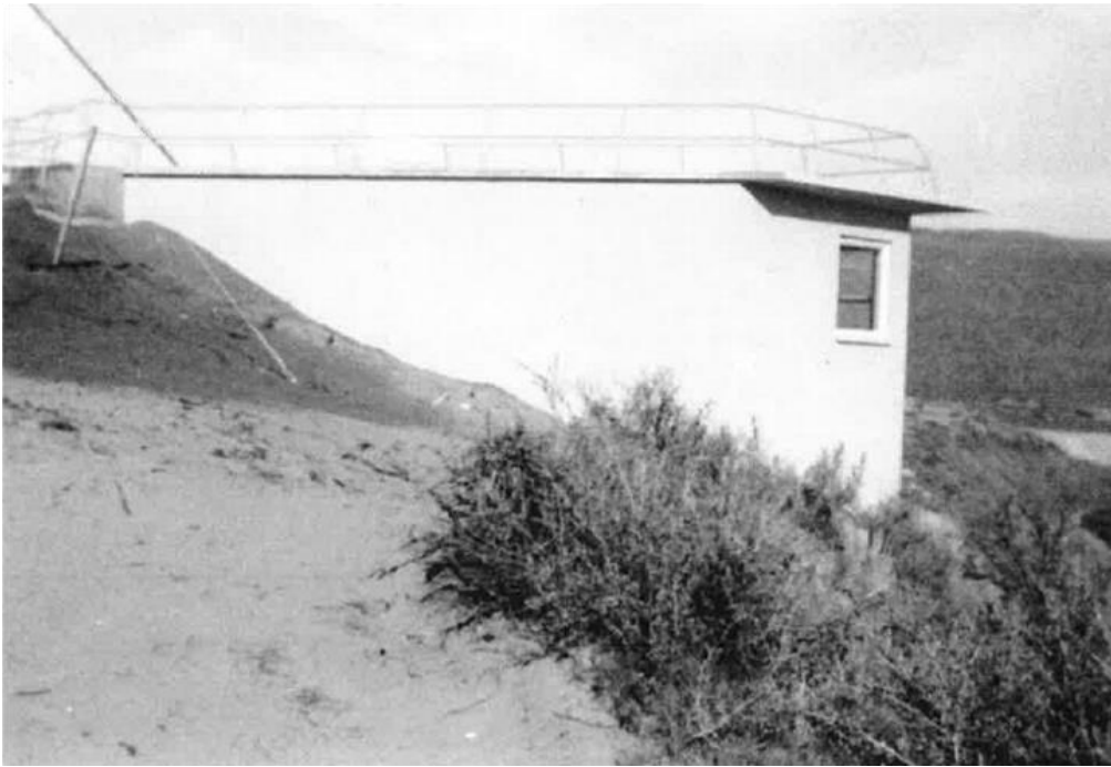
Construction photo detail showing outdoor viewing platform above living quarters. Looking north. Photographer: Unknown, obtained from Marsha Crawford Hart, c.1960
