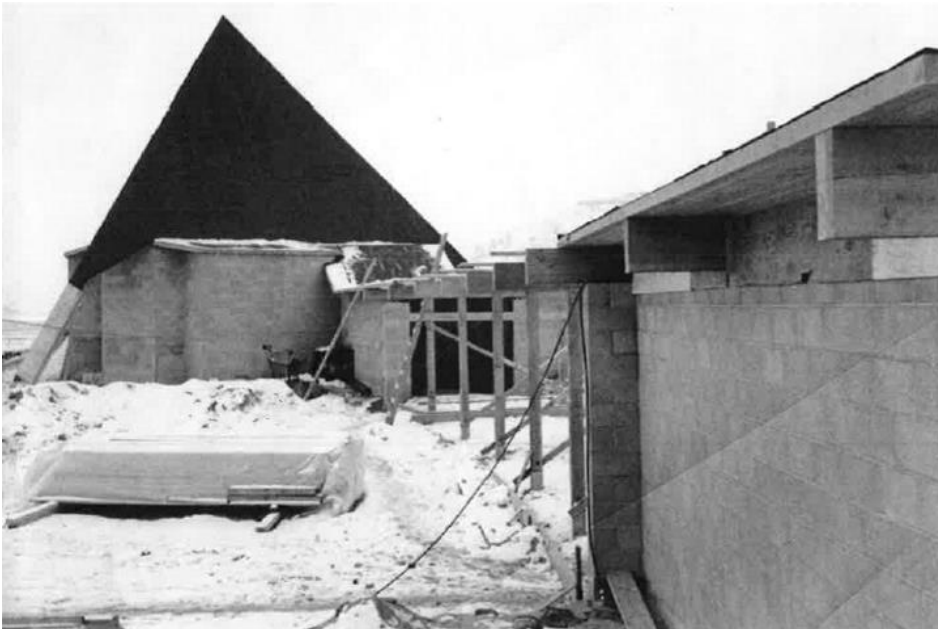
Construction photo. Comfort station is on the right, connected to the main building by a slight curved breezeway. Looking west. Photographer: Unknown, obtained from Marsha Crawford Hart, c.1960
