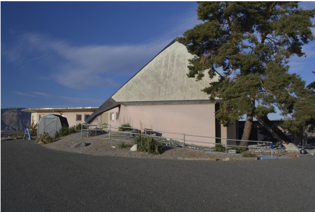
Looking southeast towards the back entrance. The A.D.A access ramp was added at an unknown date.
