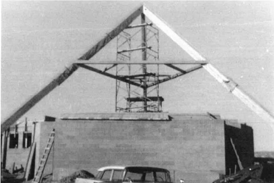
Construction photo. Pyramidal roof structure over main gallery space. Photographer: Unknown, obtained from Marsha Crawford Hart, c.1960
