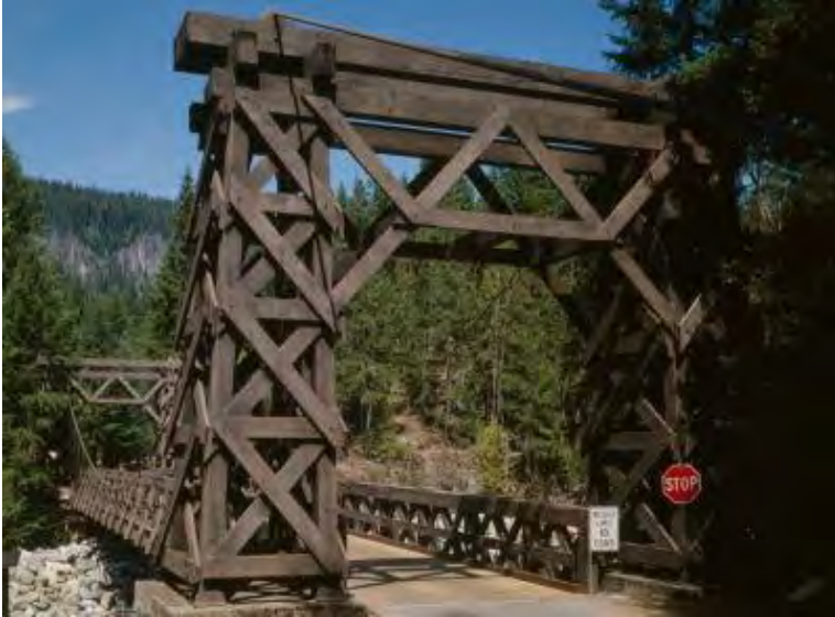
Nisqually River Suspension Bridge, Mt. Rainier National Park at Longmire – 1924 (rebuilt 2005) Photo from Historic American Engineering Record, Library of Congress
