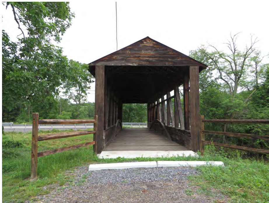
Photo 2: Cuppett's Covered Bridge looking W. Photo by AECOM, on file at PA SHPO
