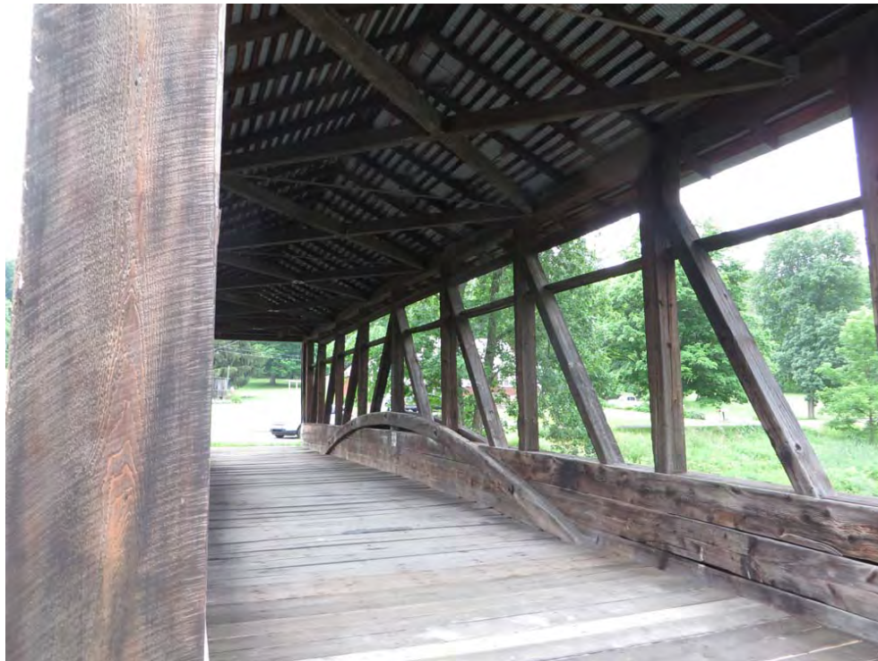
Photo 5: Cuppett's Covered Bridge interior detail. Photo by AECOM, on file at PA SHPO
