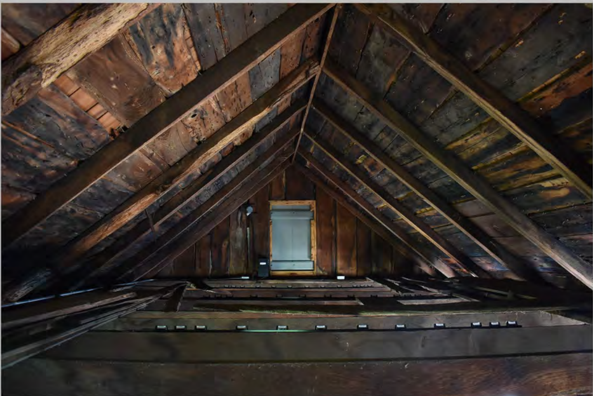
6. Interior view of the first floor of the Olney Cook Artisan Shop showing roof framing, looking northeast from southwest wall.
