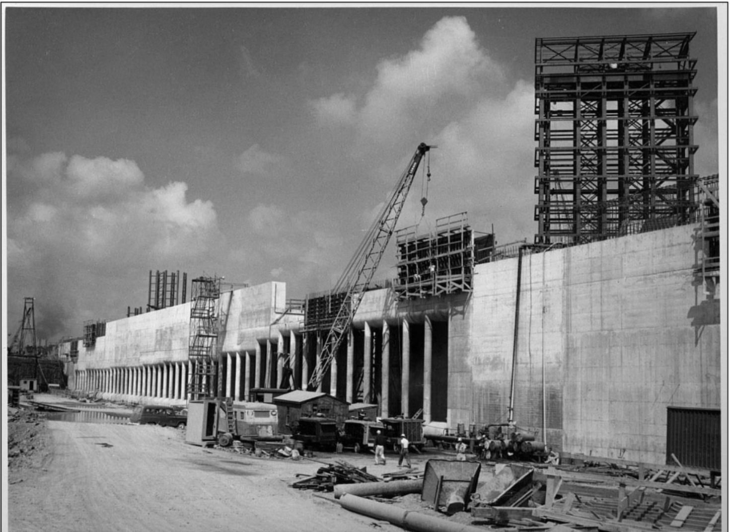
PA7-14633 NIAGARA POWER PROJECT, WATERWAYS-INTAKE. General status view looking northwesterly along face of Intake #2. Structural steel of Intake Gate Structure #1 appears at top right.
