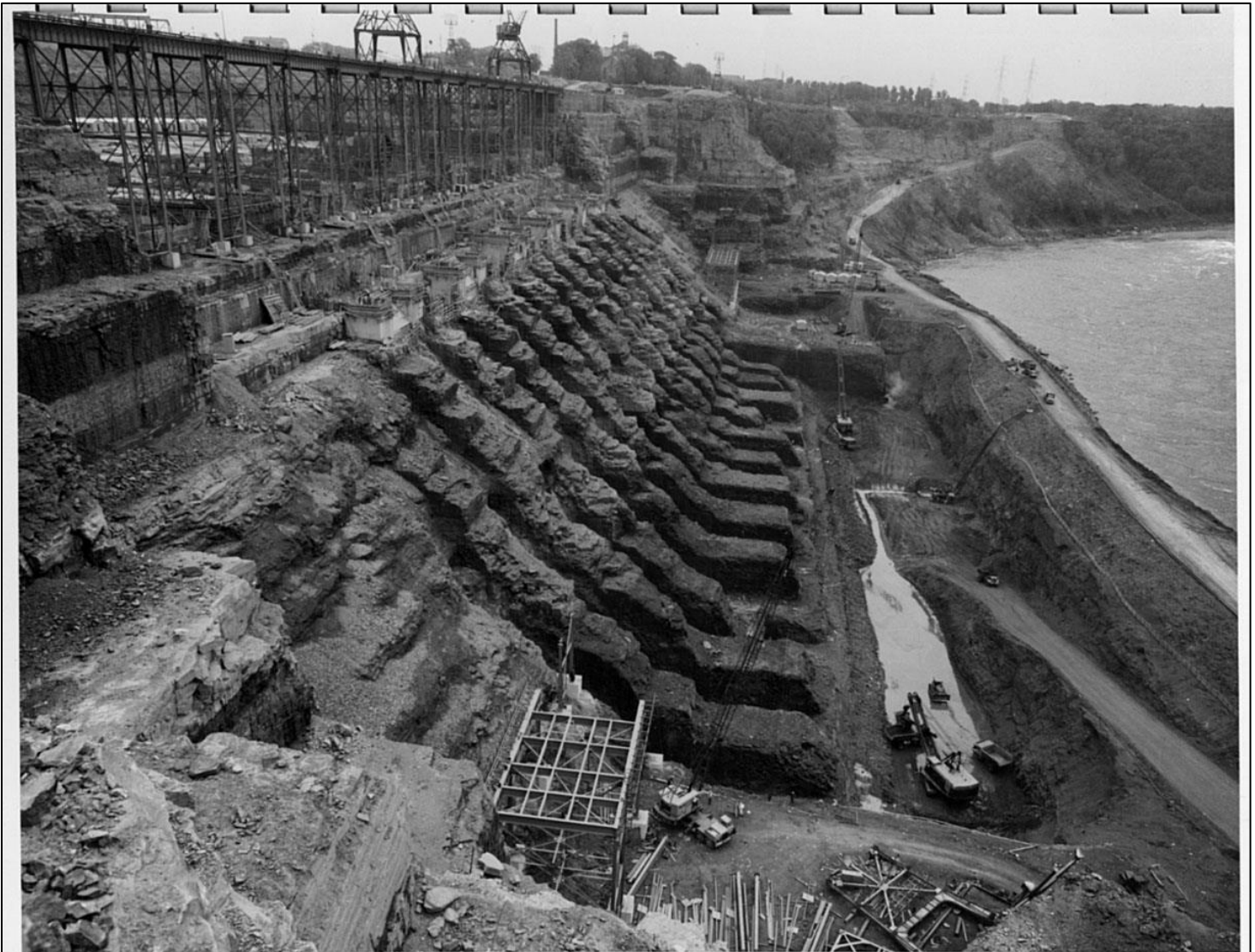
PAT-7037 NIAGARA POWER PROJECT. NIAGARA GENERATING PLANT. GENERAL VIEW OF PLANT SITE LOOKING SOUTH. LOWER GANTRY CRANE TRESTLE UNDER CONSTRUCTION IN FOREGROUND, WHILE FINAL EXCAVATION NEARS COMPLETION IN DRAFT TUBE AREA. POWER AUTHORITY-STATE OF NEW YORK UHL, HALL & RICH-ENGINEERS MAY 21, 1959
