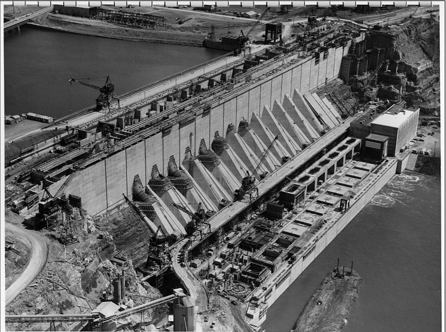
PA7-18092 NIAGARA POWER PROJECT. ROBERT MOSES NIAGARA POWER PLANT. First five penstocks are completely encased, first four units are in operation and removal of tailrace cofferdam is 75% complete as seen in this aerial view looking southeast. POWER AUTHORITY-STATE OF NEW YORK UHL, HALL & RICH, ENGINEERS May 20, 1961
