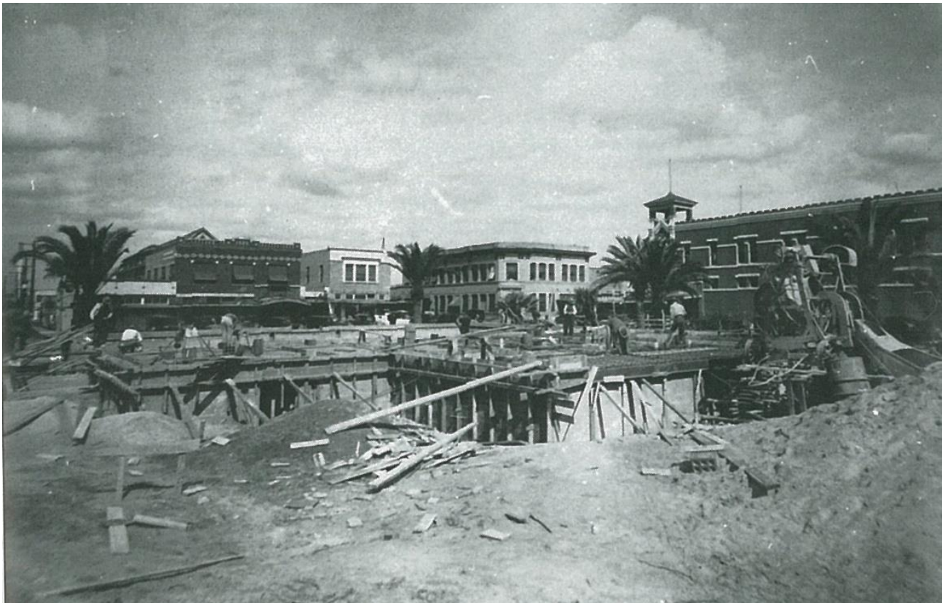
View of Caesar Park looking northeast during the construction of the new US Post Office around 1935. Source: Kingsville, crediting South Texas Archives, Texas A&M University-Kingsville.
