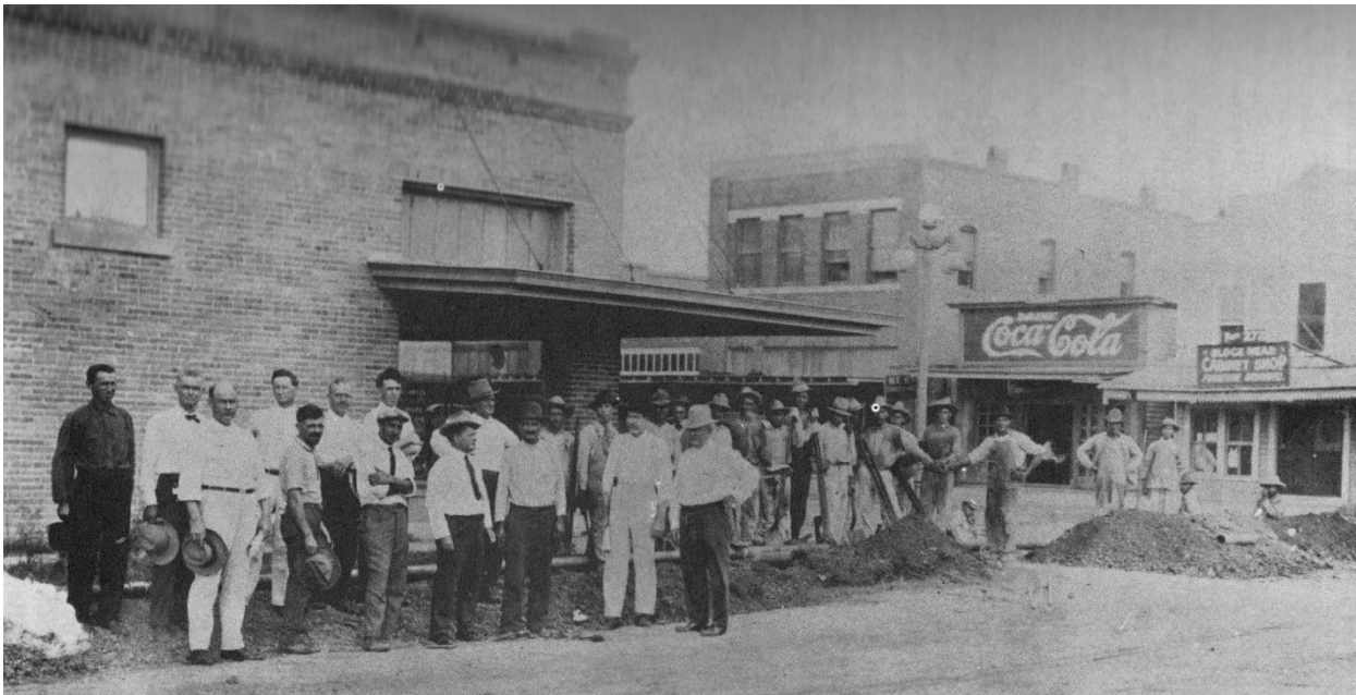
(Above) A group of men pose at the corner of South 7th Street and East Kleberg Avenue during the laying of the natural gas pipe line in September 1920. Source: Kleberg County, Texas, crediting Charles S. Flato III.
