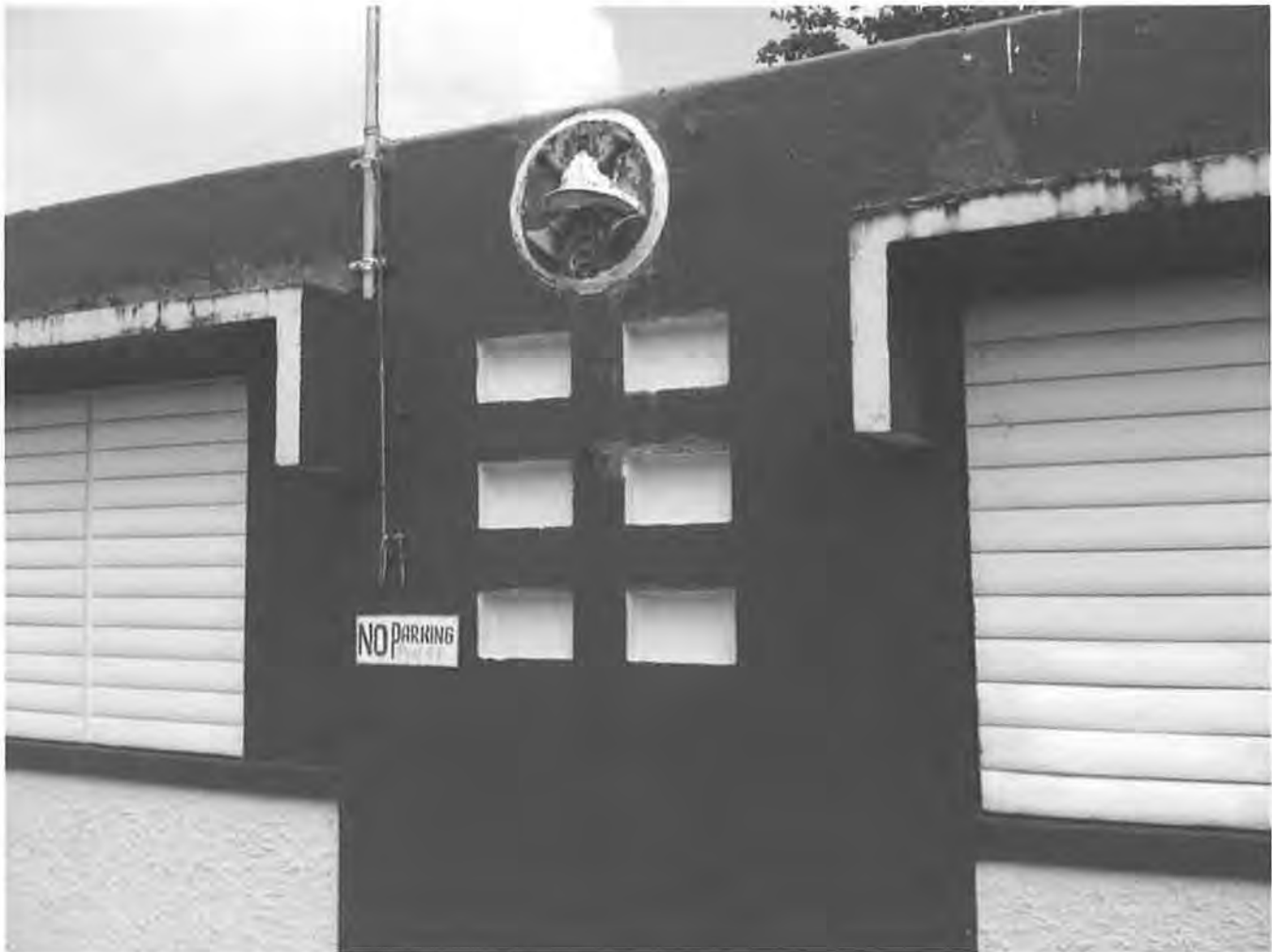
FIG. 4: Yabucoa Fire Station detail view, looking northwest, in Yabucoa, Puerto Rico. Six small, square-shaped openings divided into two columns, used to provide light for its interior spaces through glass panes. six small, square-shaped openings divided into two columns, used to provide light for its interior spaces through glass panes. Photo: Guillermo Marrero, June 10, 2012.
