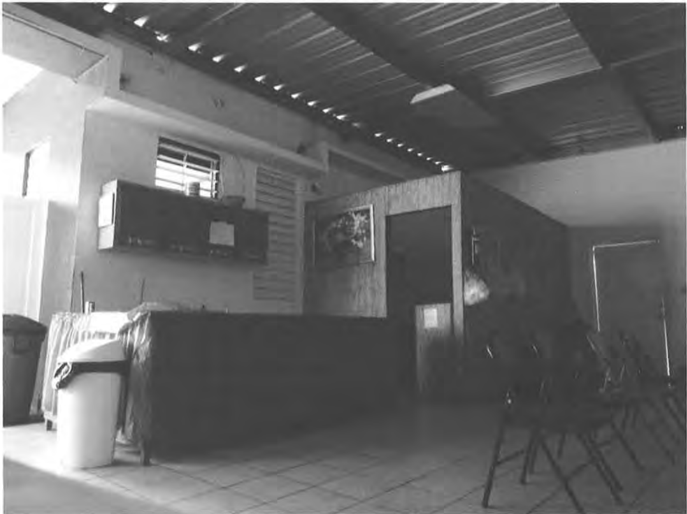
FIG. 9: Yabucoa Fire Station east elevations, looking west, in Yabucoa, Puerto Rico. The area also includes a small kitchenette behind paneled divider and attached to the back of the former fire station. Photo: Guillermo Marrero, June 10, 2012.
