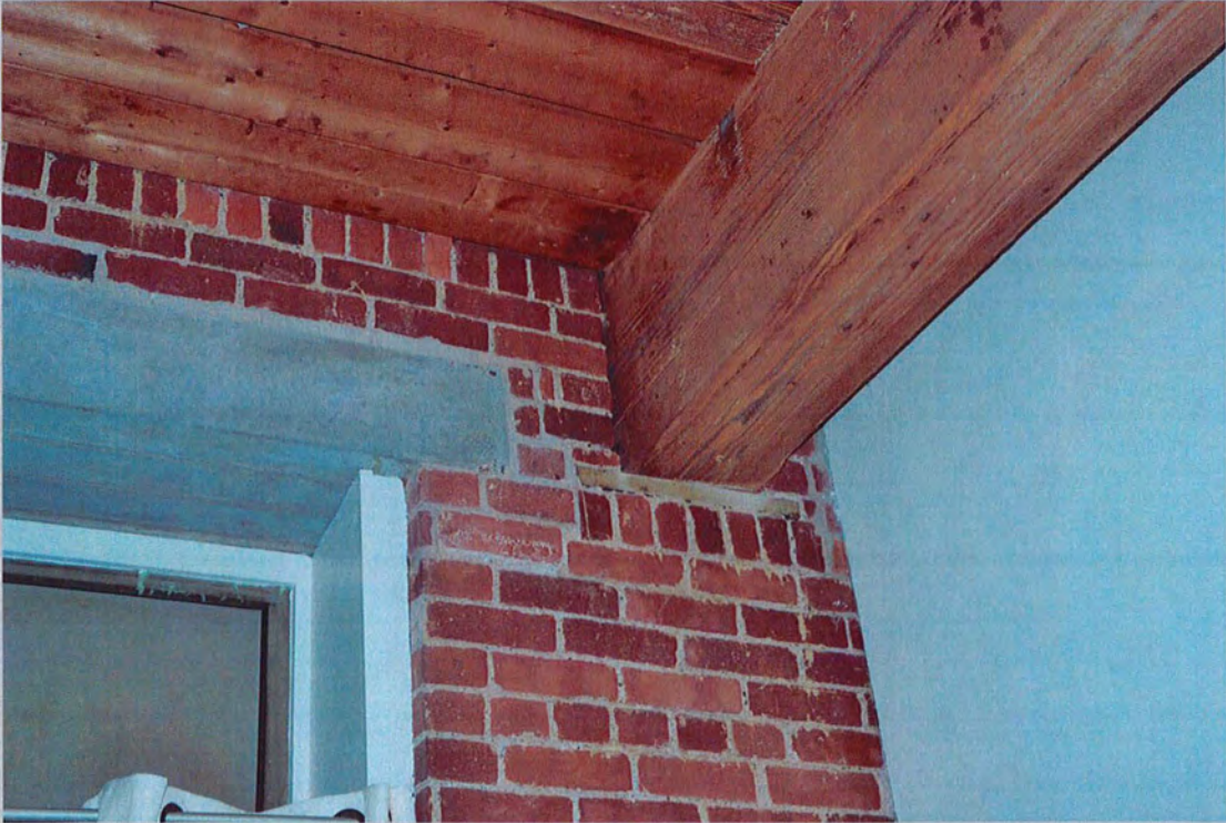
23. View northeast, unit ceiling detail showing wood beam set into pocket within exterior masonry wall (Feb. 2018).
