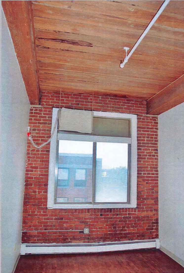
19. View south, typical residential unit showing exposed brick wall, full height ceiling and exposed wood decking – dark sugar residue visible at top left of photo along decking (Feb. 2018).
