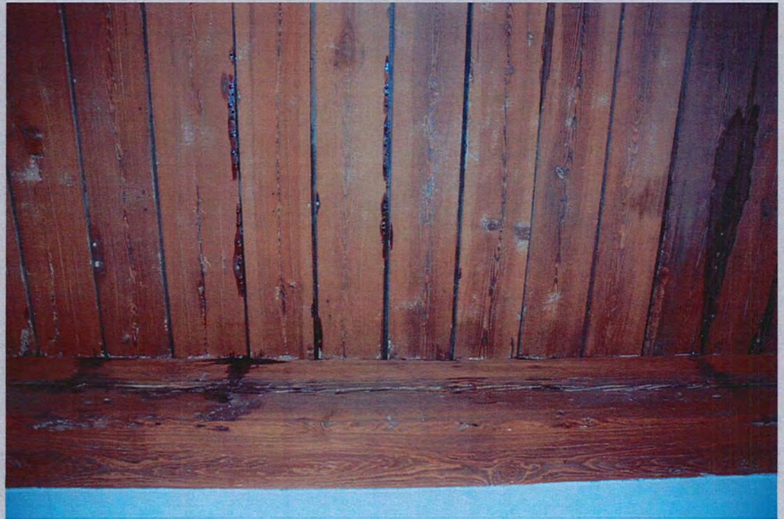
22. View west, unit ceiling detail revealing exposed wood decking – dark sugar residue visible (Feb. 2018).
