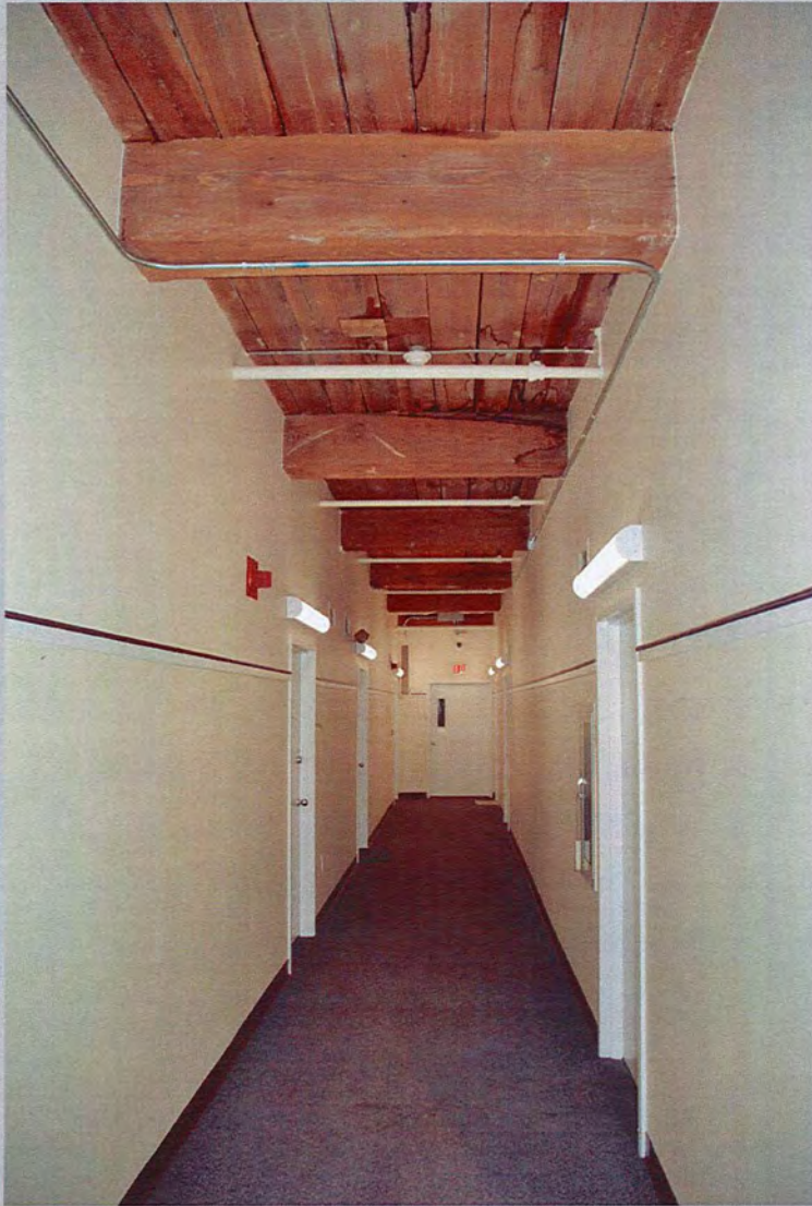
15. View west, typical hallway showing full height ceiling and exposed wood decking – dark sugar residue visible in foreground and at top center of photo (Feb. 2018).
