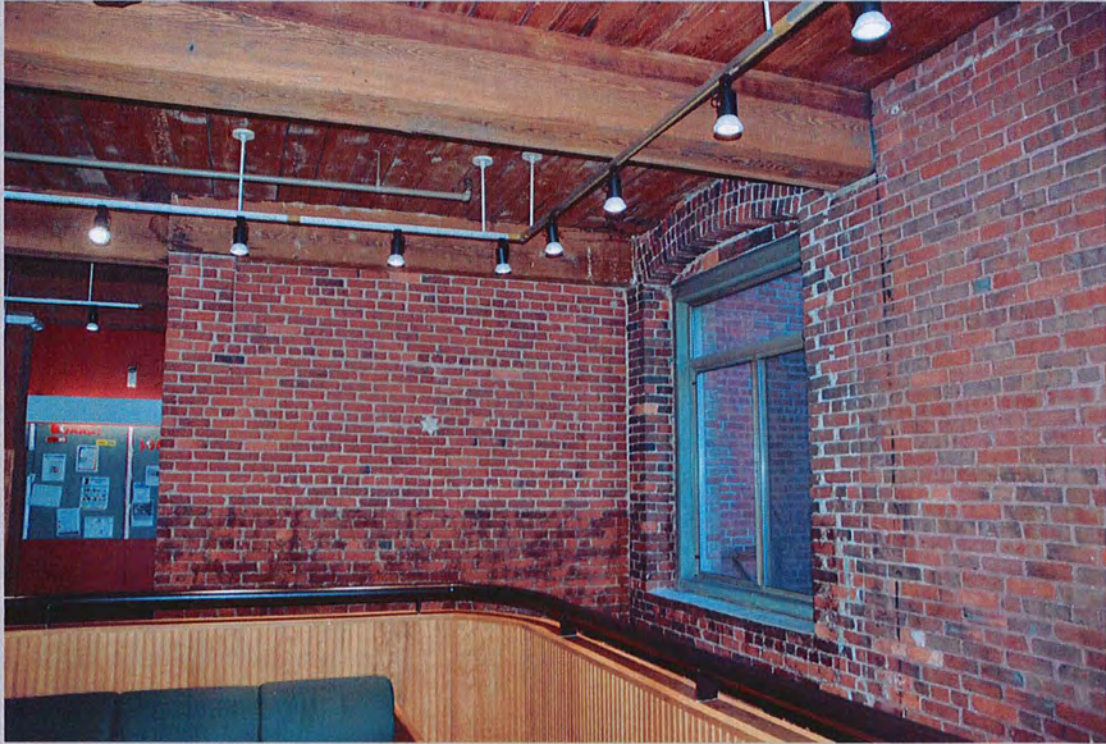
11. View northwest of lobby window with segmental arch opening and exposed brick walls and decking (Feb. 2018).
