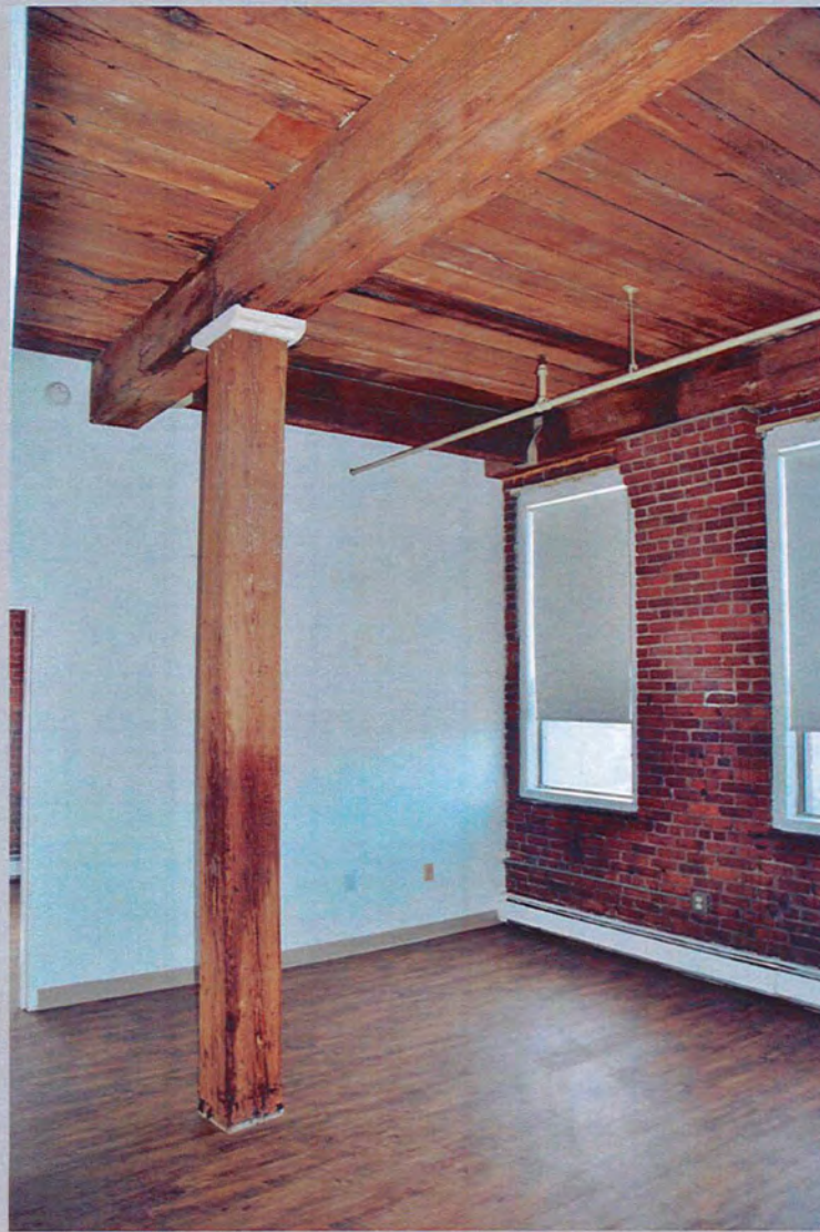
18. View southwest, typical residential unit showing corbelled brick wall, square wood column with metal cap, full height ceiling and exposed wood decking – dark sugar residue visible along I-beam and decking at top right of photo (Feb. 2018).
