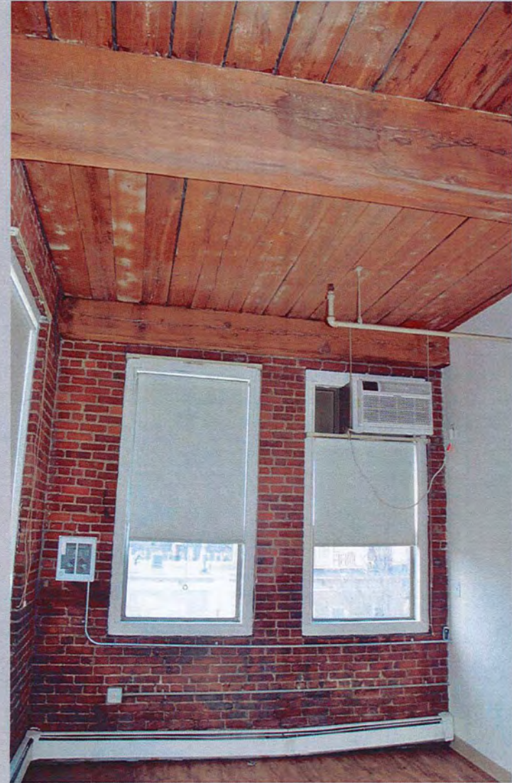
20. View east, typical residential unit showing exposed brick wall, full height ceiling and exposed wood decking – dark sugar residue visible on front of I-beam in foreground (Feb. 2018).
