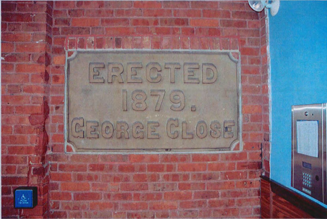
9. View south of second date stone set into the vestibule exterior brick wall - raised cast-stone lettering reads "ERECTED 1879. GEORGE CLOSE" (Feb. 2018).
