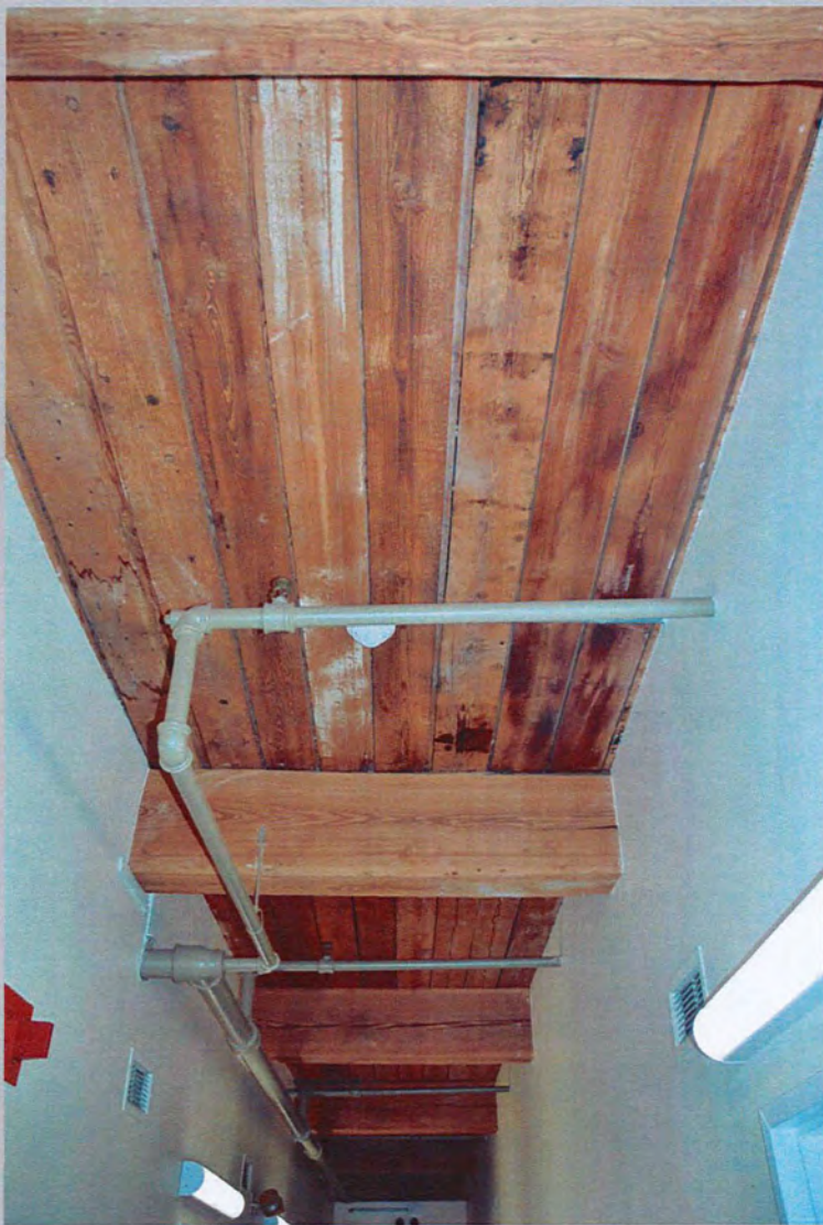
17. View west, typical hallway showing full height ceiling and exposed wood decking – dark sugar residue visible in foreground and center of photo (Feb. 2018).
