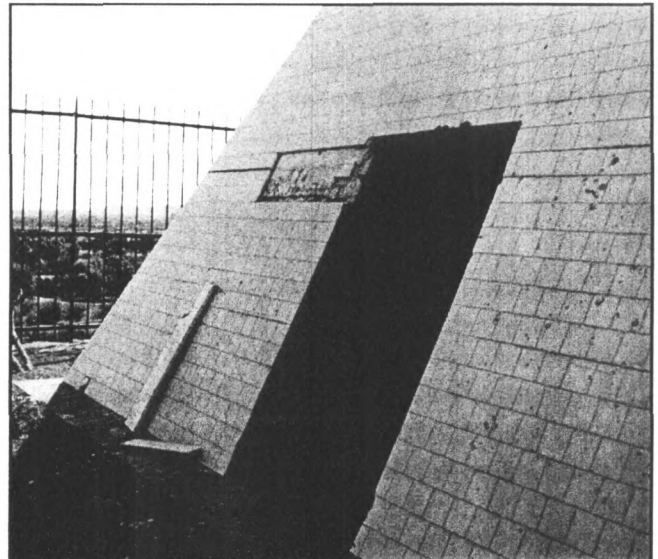
View to the south/southwest of exposed, original tile work adjacent to tomb's door. Pitting is apparent in newer tile surface at right. Sept., 2007
