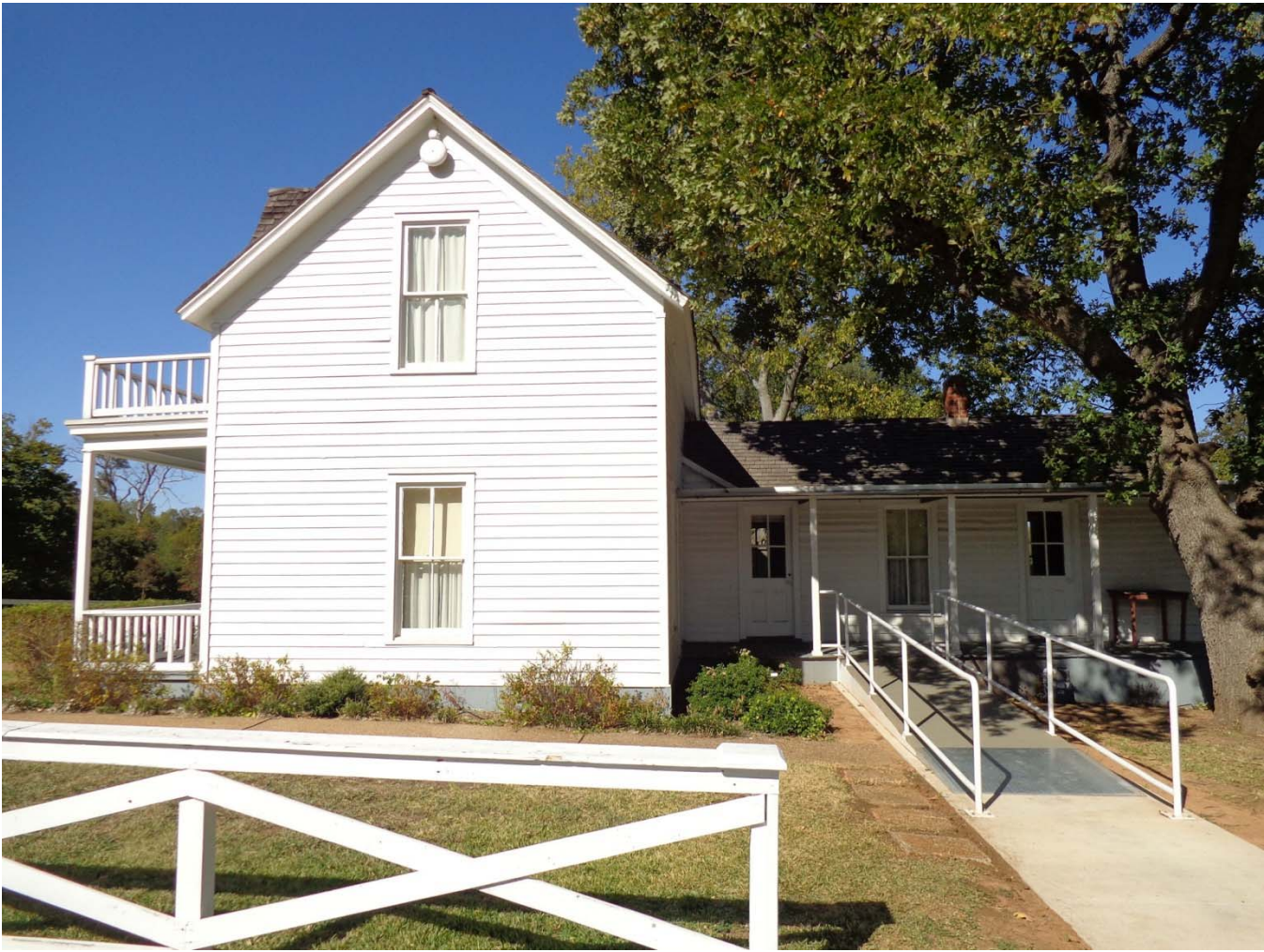
TX_Grayson County_Eisenhower Birthplace_0008 South elevation (gable end) of main house, south elevation of rear ell; view south
