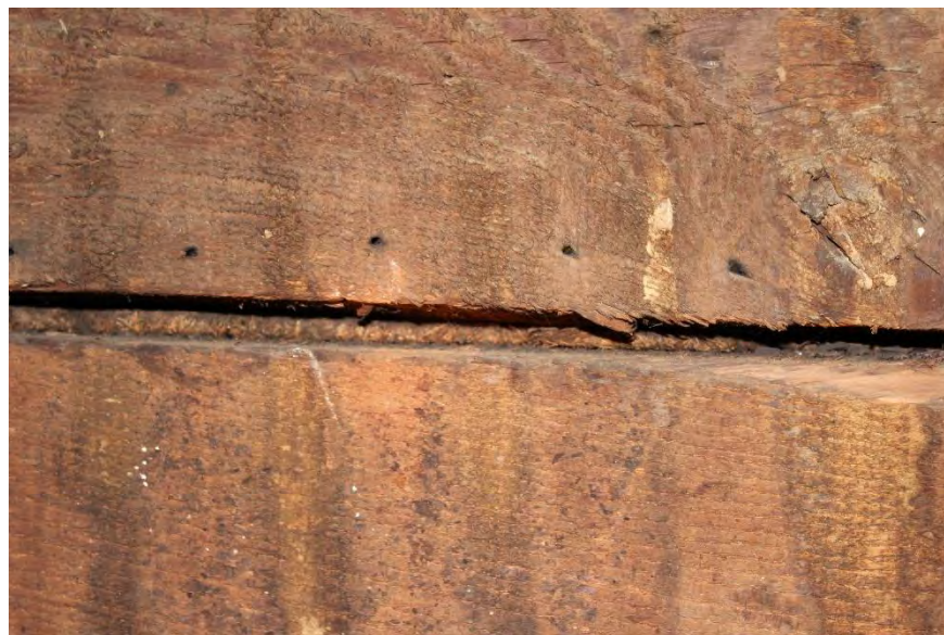
Photo 6: Interior, Original Section, 1 st floor, east wall, detail of oakum chinking between planks.
