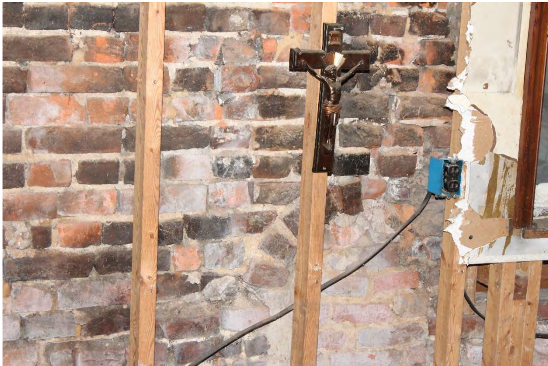
Photo 14: Interior, East Addition, north wall, detail of remnant brick arch of bakeoven aperture.
