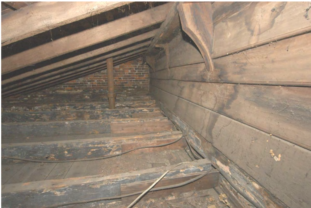
Photo 12: Interior, segment at top of east wall of Original Section where original exterior wall and cornice fabric is preserved, concealed by East Addition ceiling.
