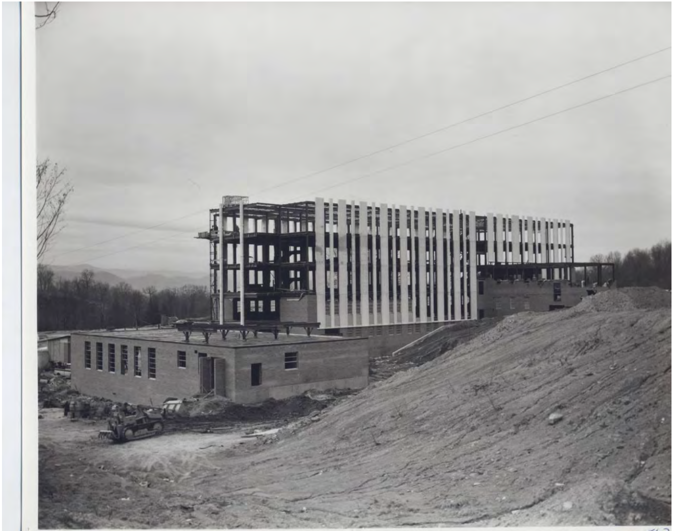
Figure 6. 1965 Photo of Smyth County Community Hospital Under Construction – Original East Wall at Left and North (Rear) Wall at Right.
