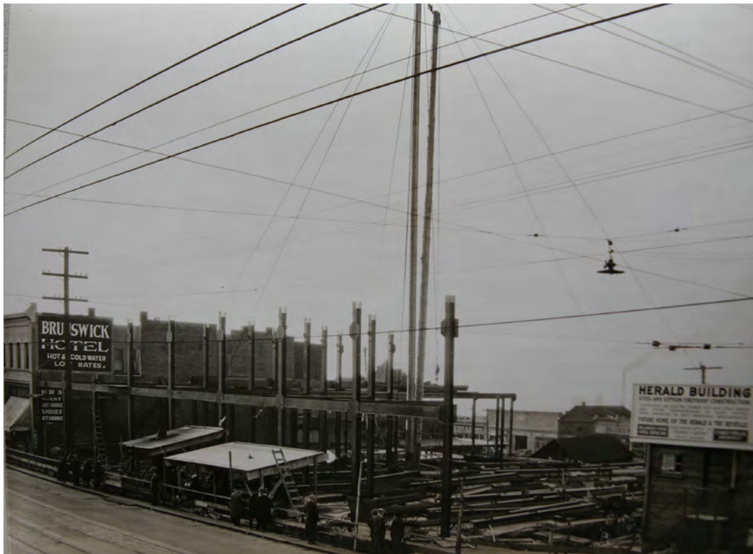
1925-26 view of steel work commencing, looking west. Source: Bellingham Herald's Jack Carver Collection, Whatcom Museum of History and Art, Bellingham, WA. Courtesy Daylight Properties.
