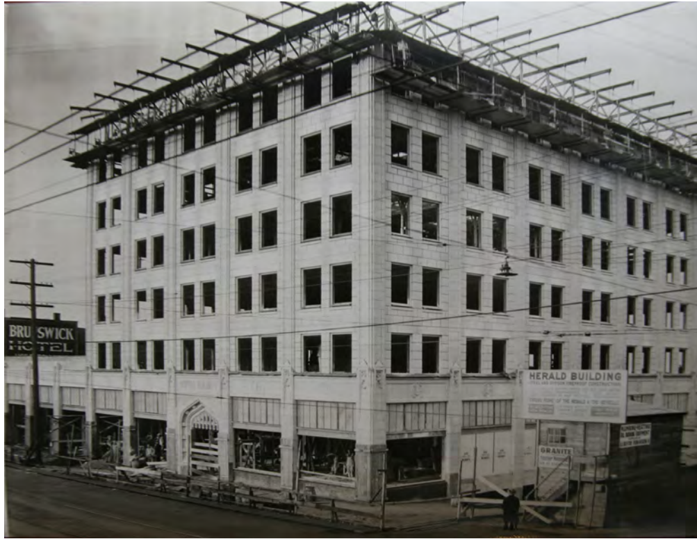
1925-26 view of terra cotta going up at the 6th floor and parapet, looking west. Source: Bellingham Herald's Jack Carver Collection, Whatcom Museum of History and Art, Bellingham, WA. Courtesy Daylight Properties.
