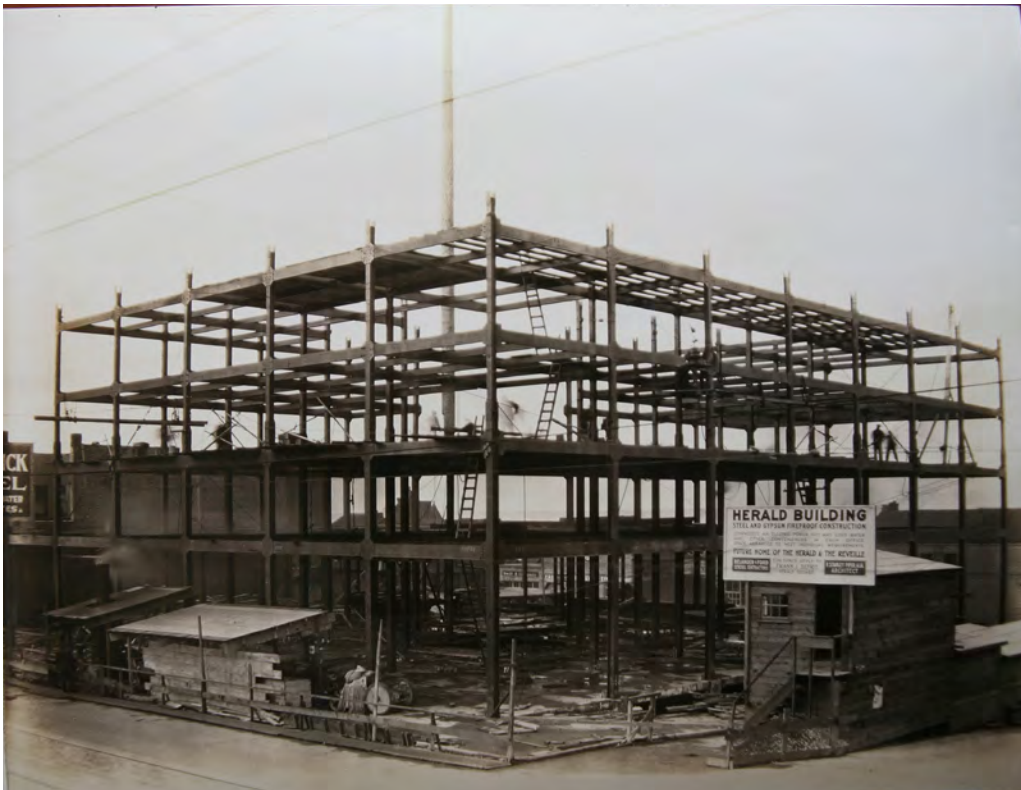
1925-26 view of steel work, looking west. Source: Bellingham Herald's Jack Carver Collection, Whatcom Museum of History and Art, Bellingham, WA. Courtesy Daylight Properties.
