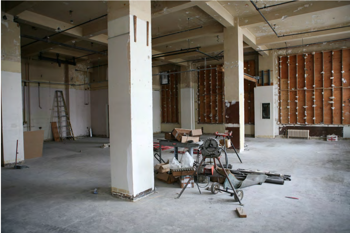
Photograph 13 of 18: Interior view of former composing room, looking west. Original bloxonend flooring still present.
