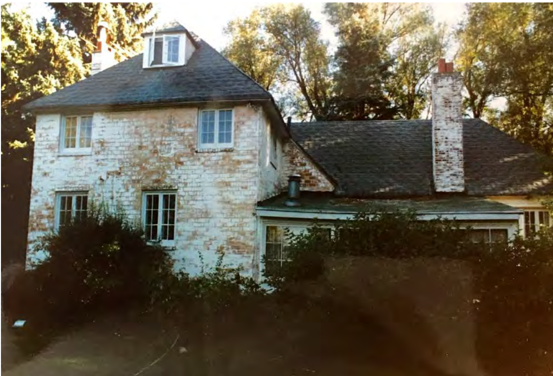
Figure 6 of 6. Photo taken in 1988, after sanding, showing the underlying lime paint.
