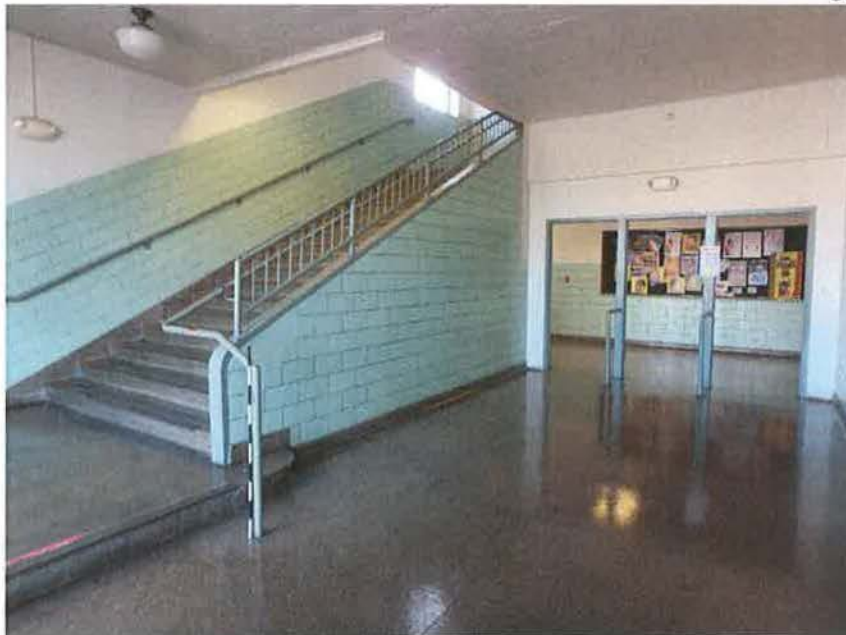
Figure 10. Overview of a foyer within the Junior High school portion (west wing) of the Dunbar School, view facing east-southeast (2018) (AZ_PimaCounty_DunbarSchool_0004).
