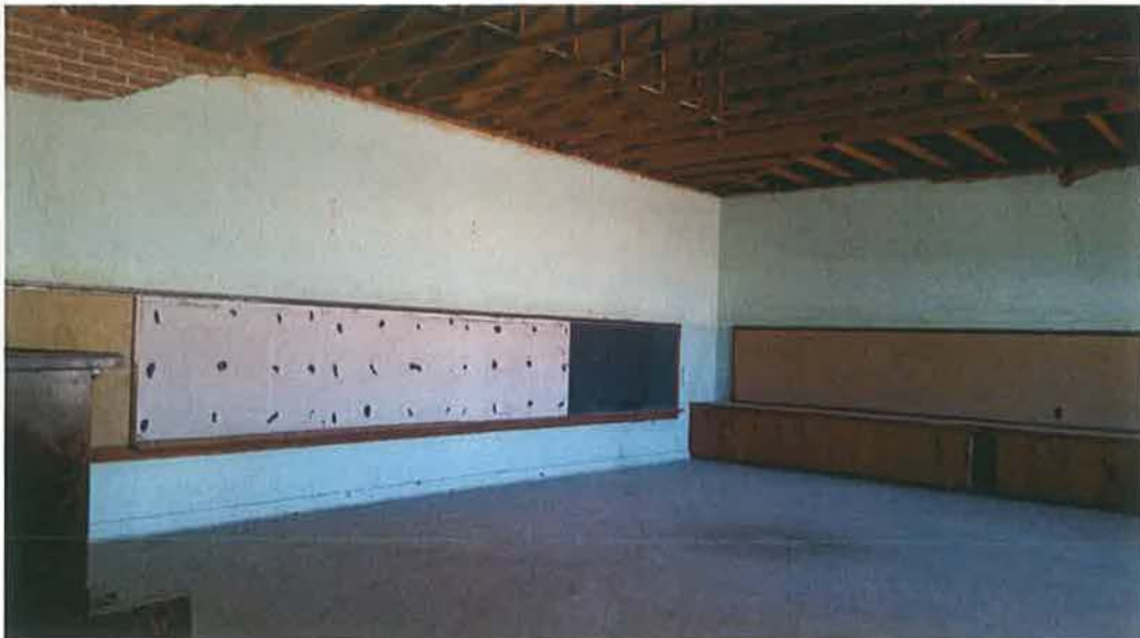
Figure 26. Detail of a classroom in the 1918–1940 portion of the school, view facing southwest (AZ_PimaCounty_DunbarSchool_0018).
