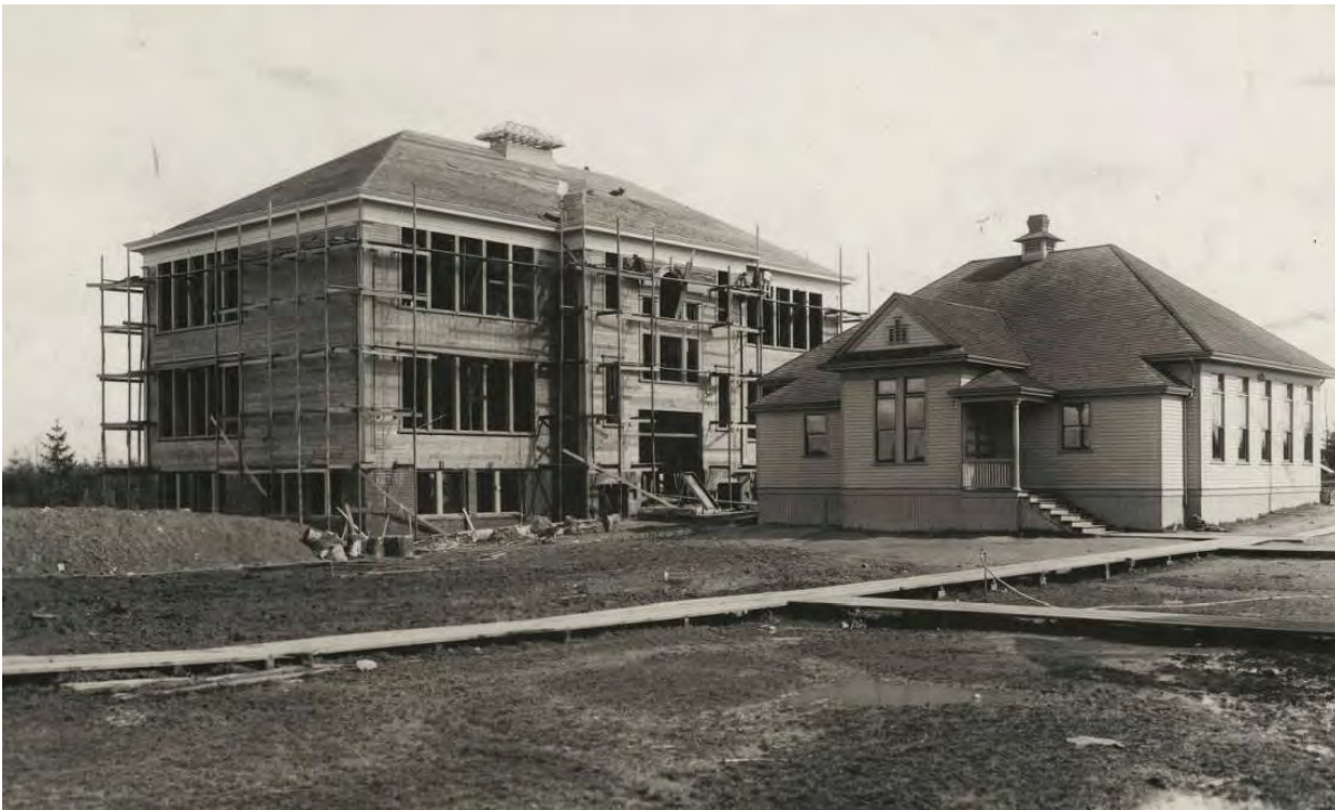
First wing of Beacon Hill School under construction – 1903-04. Two-room Beacon Hill School built in 1899 to the right. University of Washington Digital Collections
