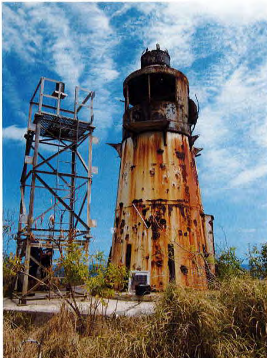
2018 Photo # 1. Exterior southwest elevation, camera facing northeast, 2018 (VI_St Croix County_Hams Bluff Light_0003).
