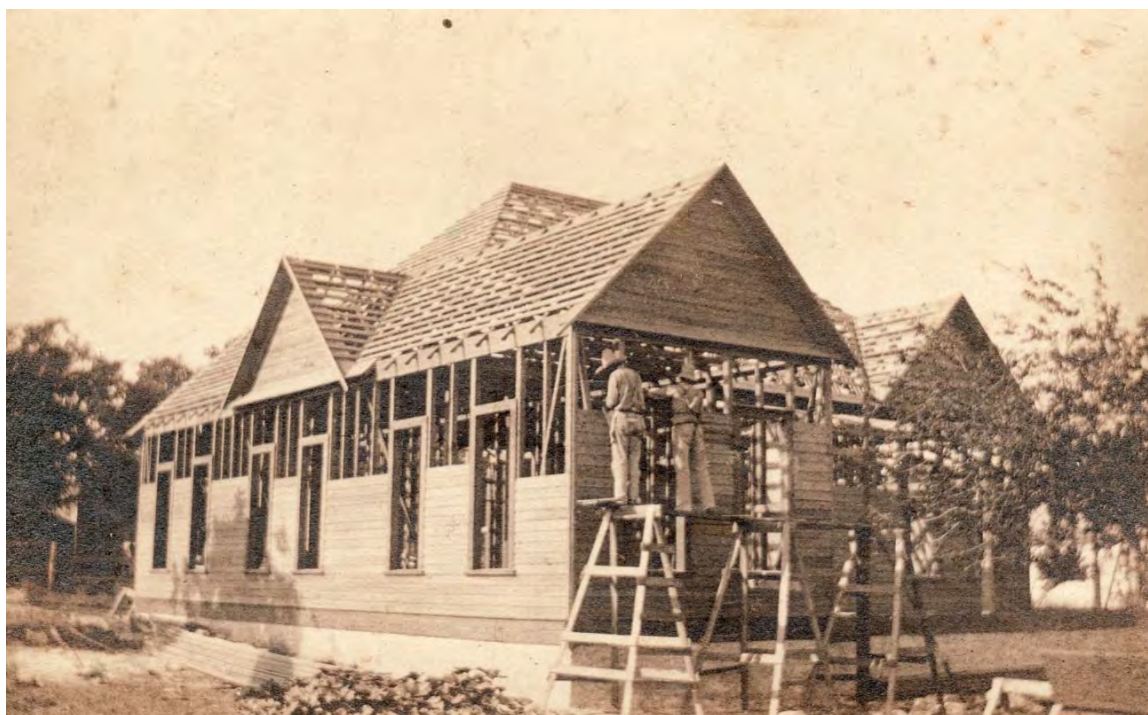
Figure 8. Ca. 1910 photograph of Hermann, Jr.'s house under construction. Source: Arnold B. Fischer Photograph Collection, courtesy of Bryan Weidner.
