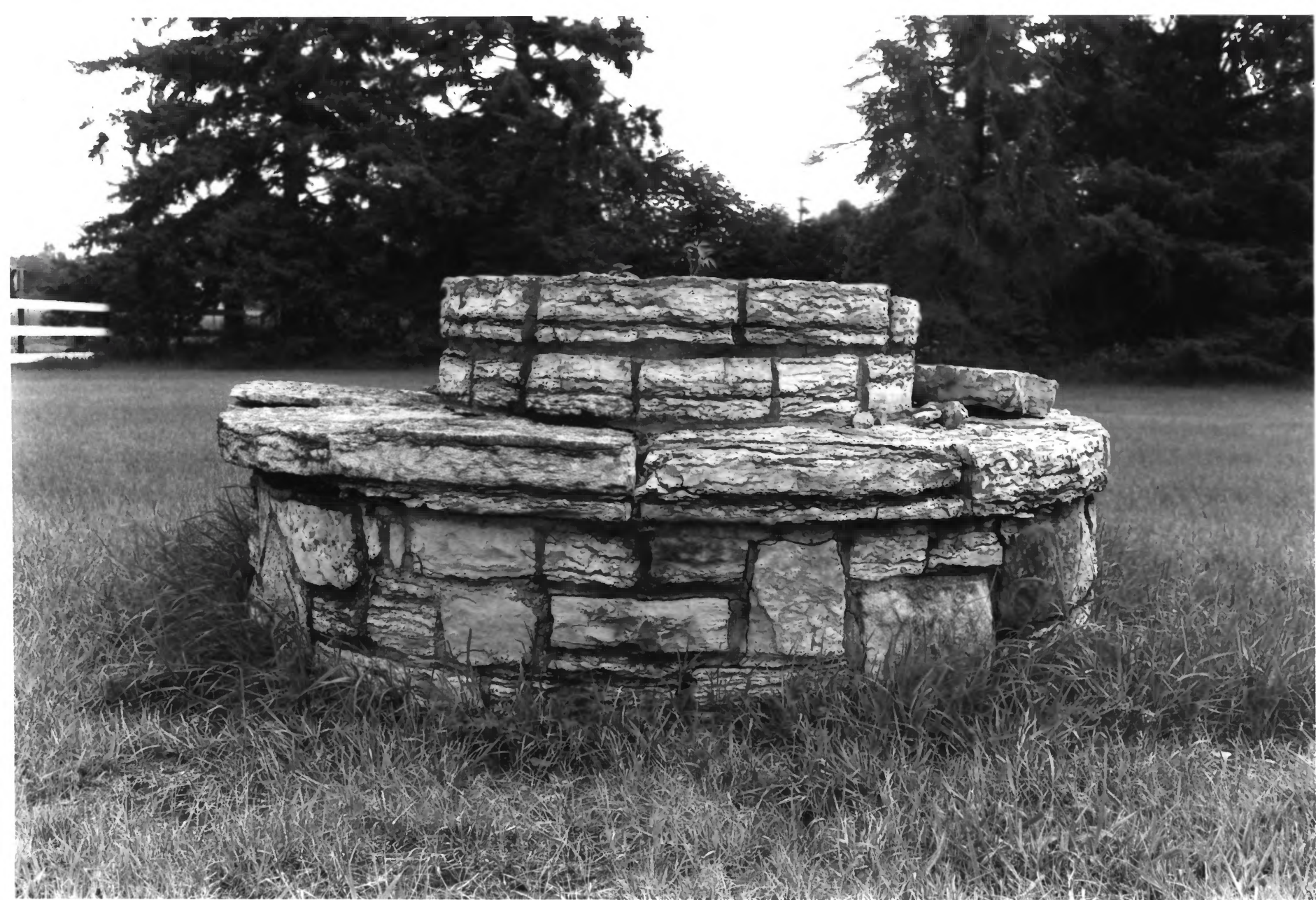
Utility Access Structure, Carlos Avery Game Farm Ham Lake vicinity, Anoka County, MN 010831 - 18A/19
