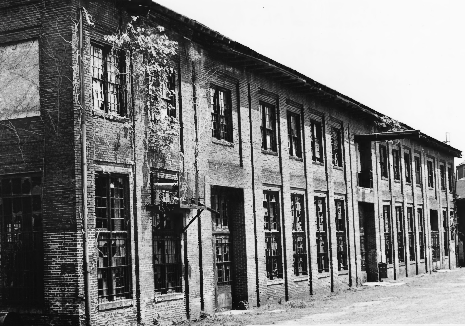
Photograph #3 B&O RAILROAD MARTINSBURG SHOPS Martinsburg, WV West facade of Machine/Woodworking Shop, looking southeast. Michael Caplinger, IHTIA, August 2001
