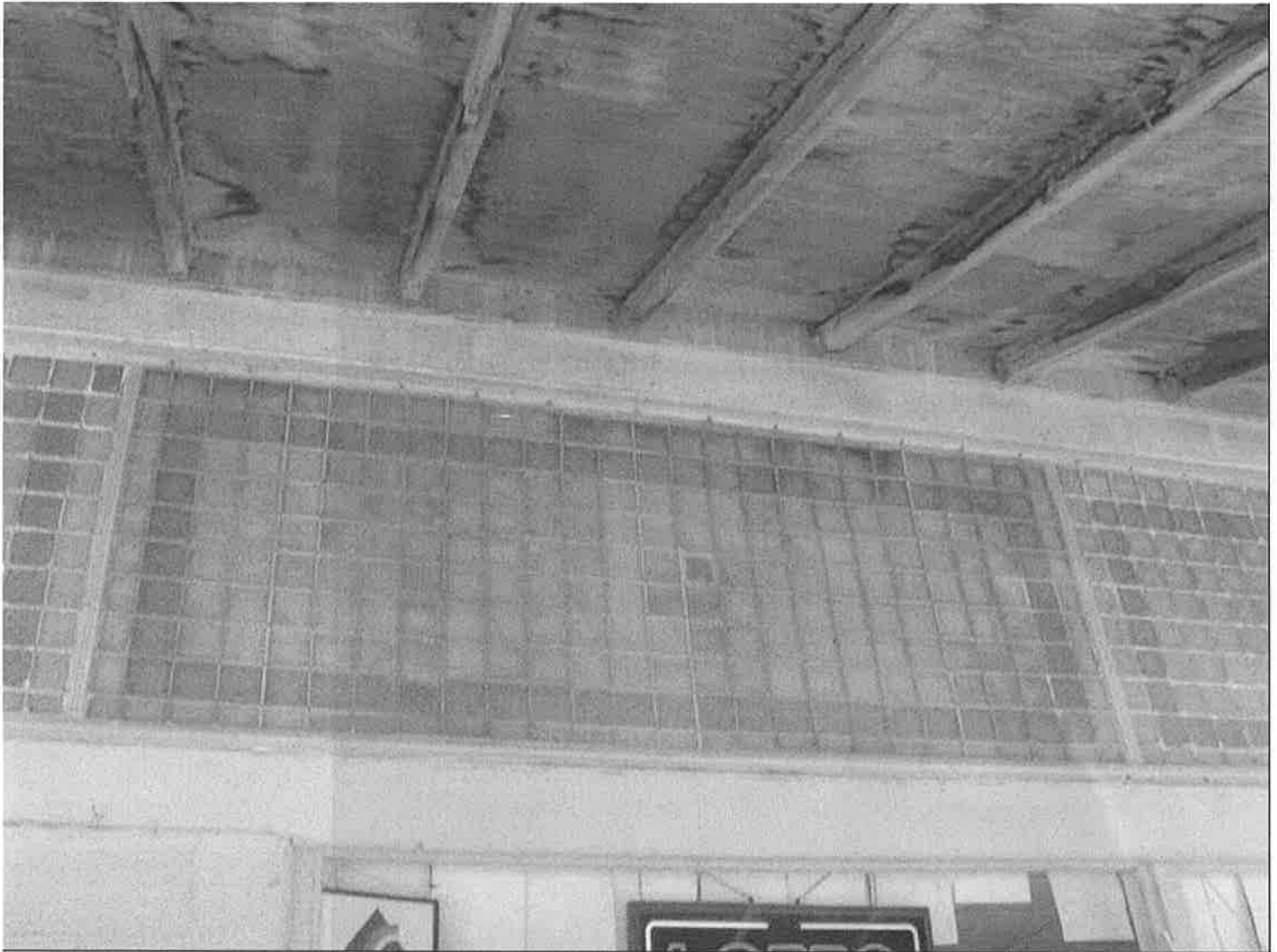
Photo 0010. Detail of Colored Block Clerestory of Kose Hall. North façade. View to the south.
