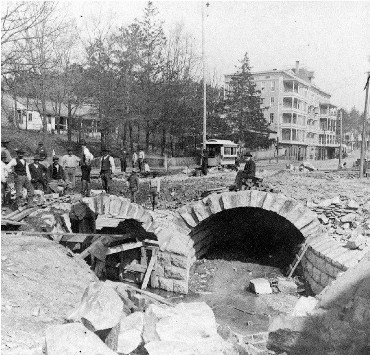
Figure 2. Construction of stone arch spanning Hot Springs Creek, c. 1884 (Garland County Historical Society Archives, Photograph Collection)
