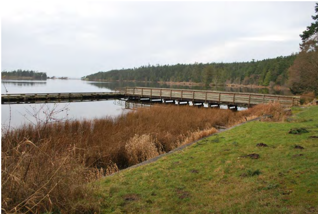
Photo 14 of 14: Cranberry Lake Dock (ID#11), view to northwest taken 12/22/2014. Top of the south section of the seawall visible adjacent to the edge of grass.
