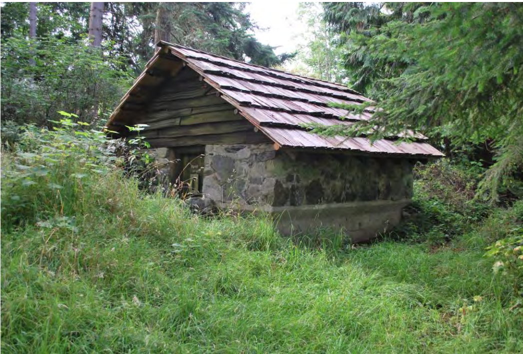
Photo 7 of 14: Pump House (ID#5), view to southeast taken 8/1/2012.
