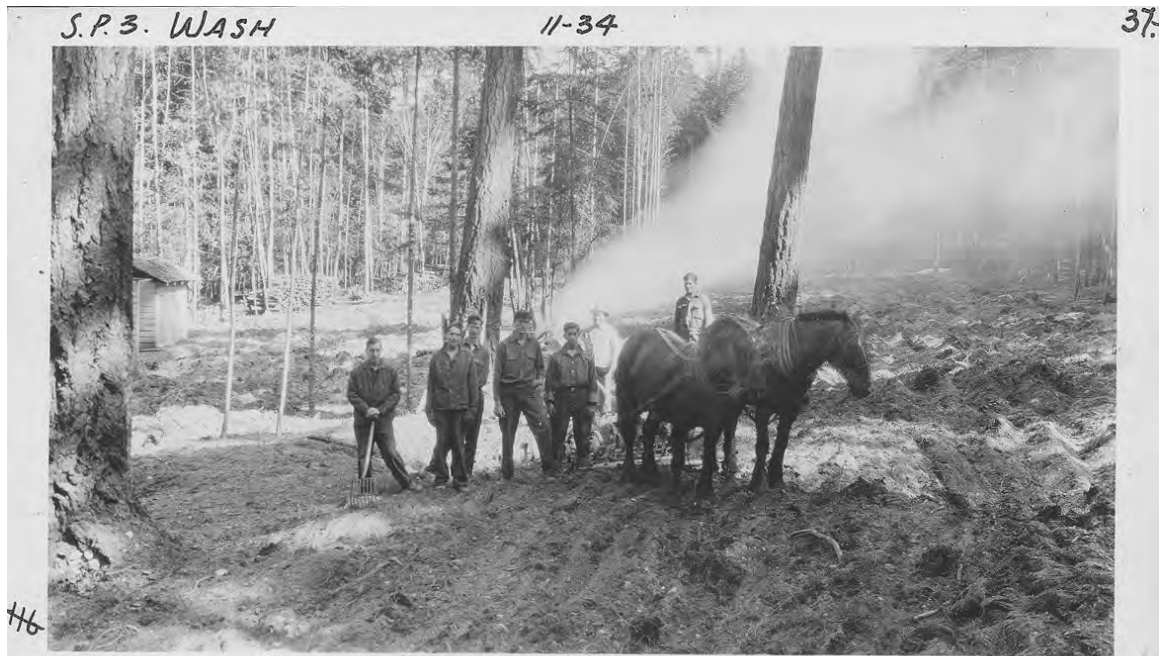
46 CLEARING PARK AREA AT CRANBERRY LAKE. Clearing prior to construction of the north portion of the parking area.
