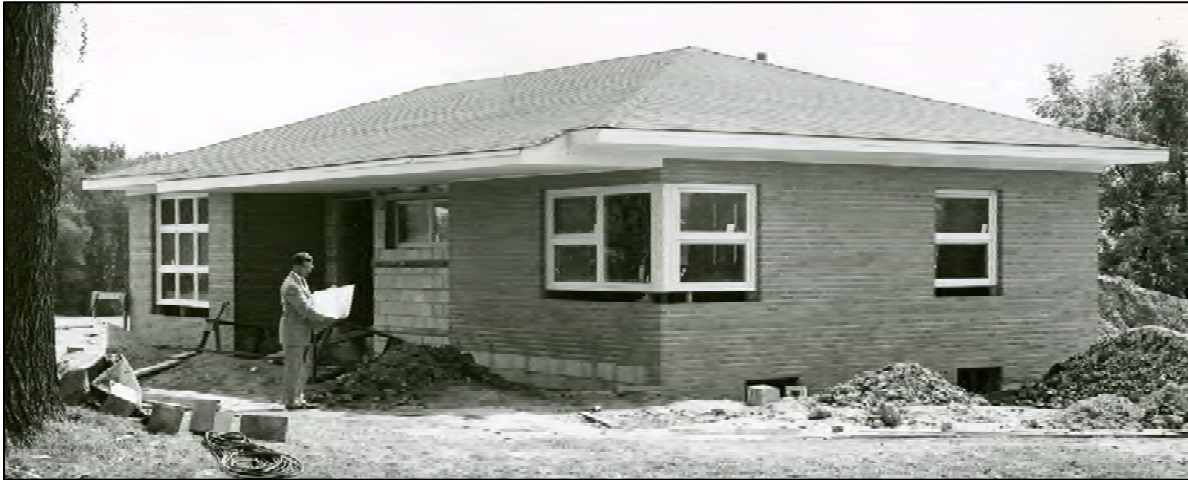
Top Left: current view of administration building. Top Right: circa 1957 photo of office building. Bottom: building under construction in 1956.
