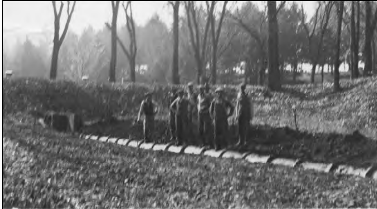
Photographs of workers in the early twentieth century installing underground vitrified pipeline in the ravine and connecting to the culvert under one of the driveways.
