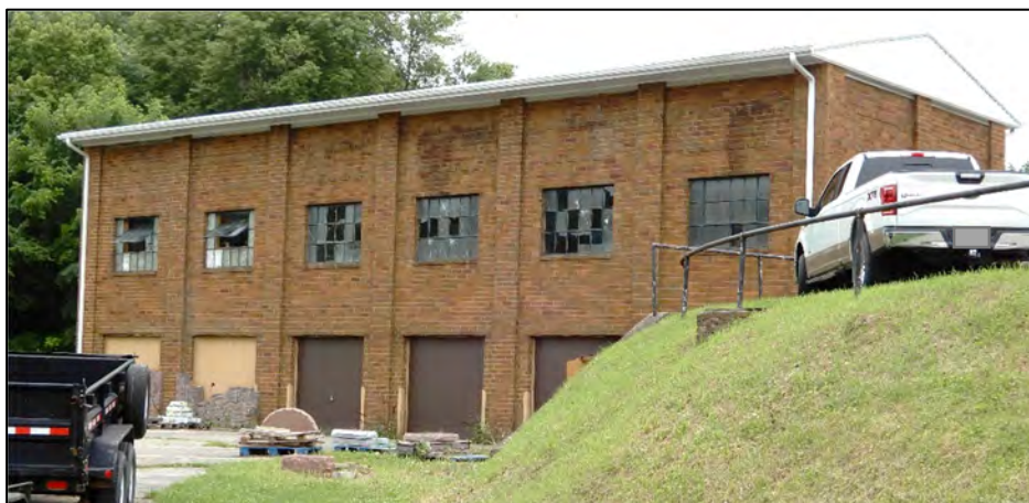
North (rear) of Service Building looking SE and taken July 17, 2021 by Tallgrass.
