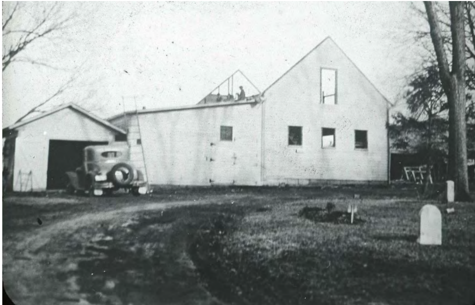
Photo of a barn being torn down to make way for the extant service building. Aspen Grove Cemetery photograph collection.
