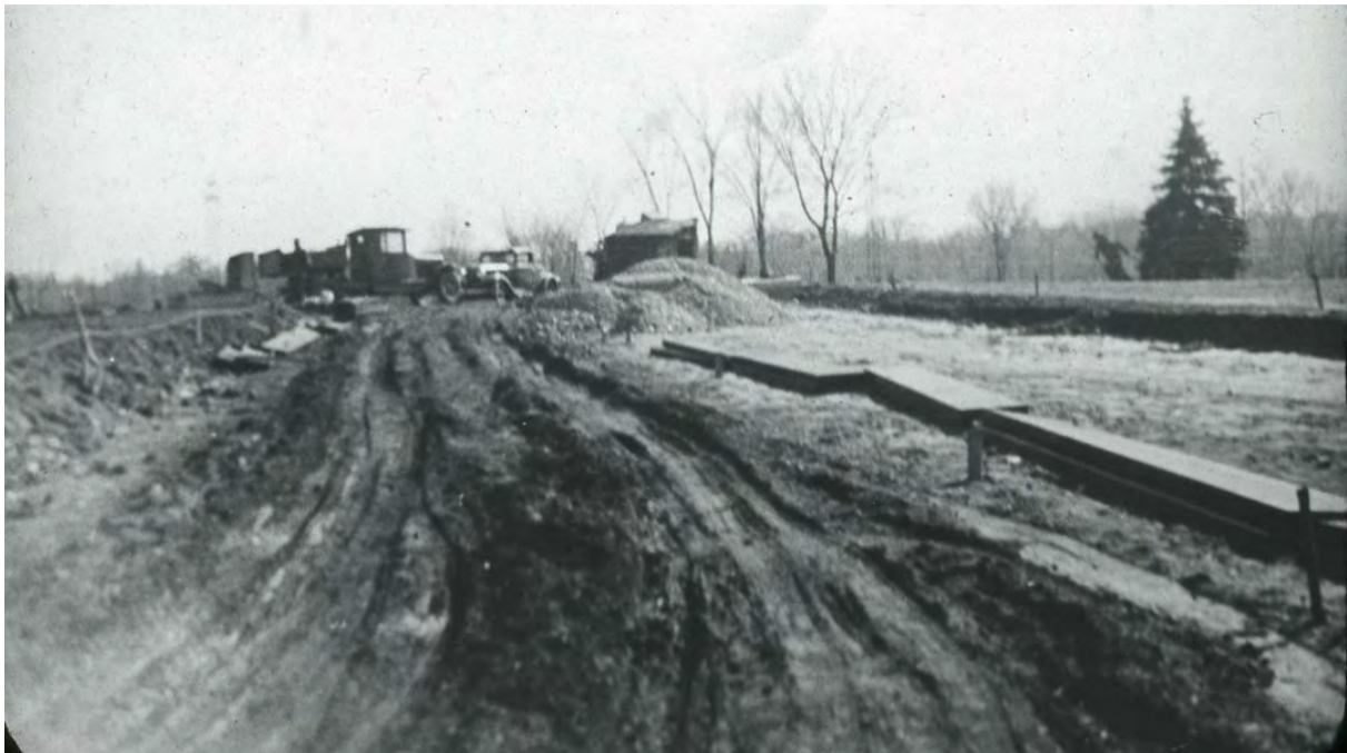
The Sunnyside Ave entrance under construction (current main entrance) in the early 1950s.
