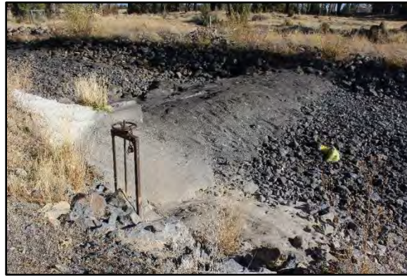
Historic lift gate assembly (Headgate #6 in Table 1) with no headwall and crude concrete check that has been built up over time. 74
