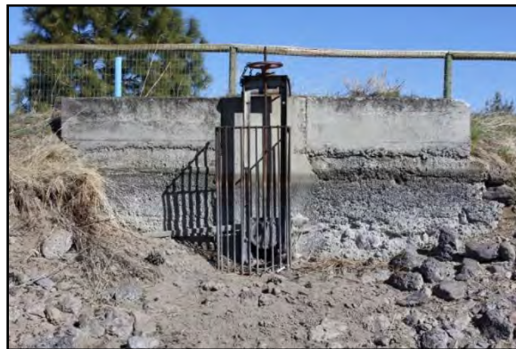
Looking north from the center of the canal bed to historic headgate, COC 8/9, near Ward Road. 76 The handmade reinforcing-bar cage keeps rocks out of the pipe. It is attached to a worn concrete headwall. The pipe serves two ditches that branch out from a weir box north of the berm (Headgate #1 in Table 1).
