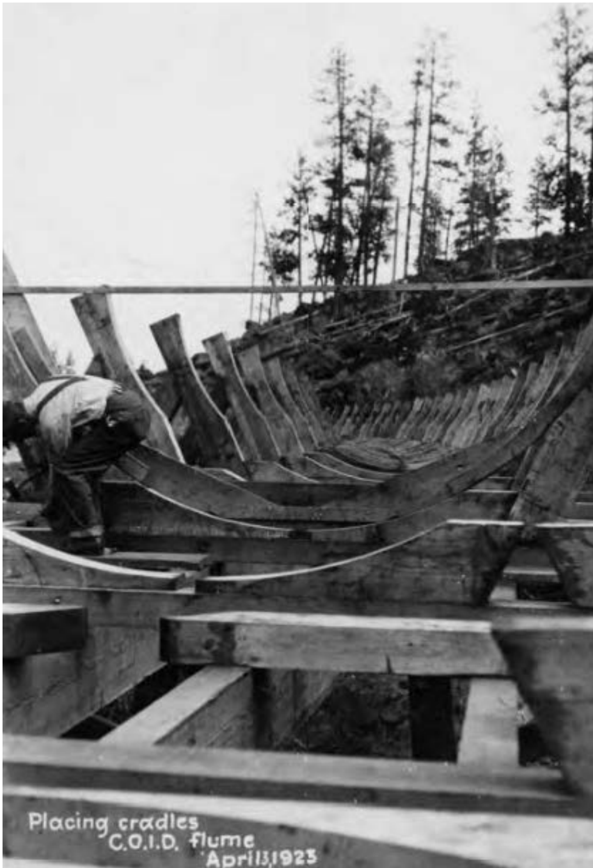
Example of a semi-circular wooden stave flume under construction within the Central Oregon Irrigation District. While not specifically the Central Oregon Canal Flume no. 2, this photo illustrates construction techniques as well as the support structure for these types of features. Photo courtesy of COID.
