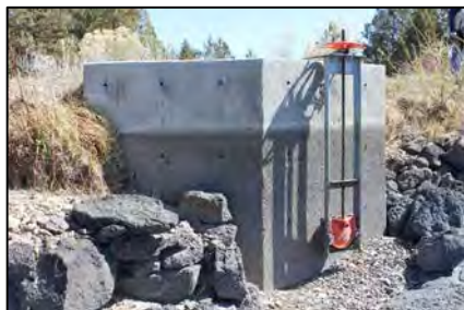
A non-historic headgate, centered on the headwall, with wing walls angled into the canal. (Headgate # 11 in Table 1.) 79
