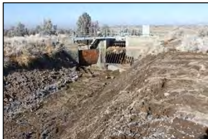
The intake structure with a trash rack to keep debris out of the steel pipe that crosses the Dry River bed. The wastewater spillway gate is on left. Photo shows recent major alterations to the canal bed and side slope. 409
