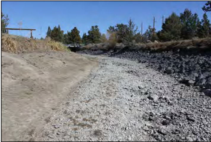
Photo 20 of 20: Looking east to Gosney Road Bridge at east end of historic district. Tall berms are on both sides, north side is silted. Canal is 59' wide and 5.5' deep.
