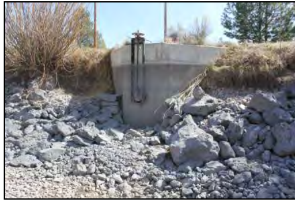
Looking south to newest headgate that delivers water through a pipe to a weir box and delivery pipe on the south side of the canal to serve a new patron, just southwest of the Gosney Road Bridge. 77
