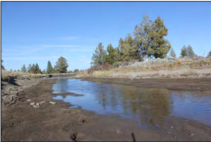
Photo 8 of 20: Heavily silted canal bed holds water year around, looking east.
