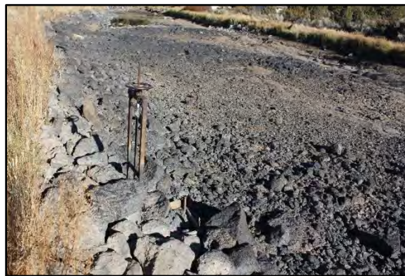
Sections of wood sit in the rocks at the base of this historic headgate. There is no headwall. In Table 1 it is Headgate #2. 75
