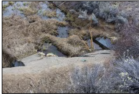
The headgates at Stearns Waste can discharge water from the canal to COID scrub land in an emergency. 67
