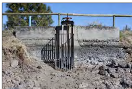
Looking north from the center of the canal bed to historic headgate, COC 8/9, near Ward Road. 77 The handmade reinforcing-bar cage keeps rocks out of the pipe. It is attached to a worn concrete headwall. The pipe serves two ditches that branch out from a weir box north of the berm. (Headgate #1 in Table 1)
