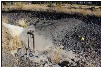
Historic lift gate assembly (Headgate #6 in Table 1) with no headwall and crude concrete check that has been built up over time. 75
