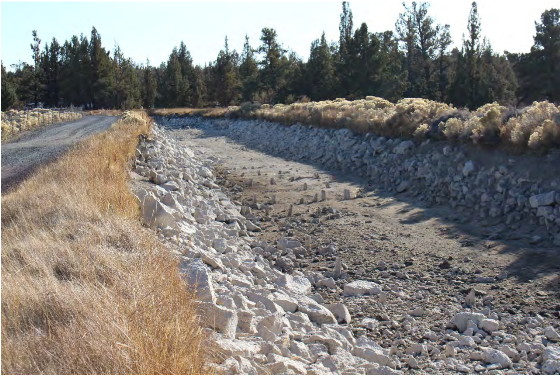
Overview of flume remnants from along the north side of canal, approx. middle of site, facing east. Ditchrider road to left. Note linear alignment of post remnants, depth and steepness of south canal wall.
