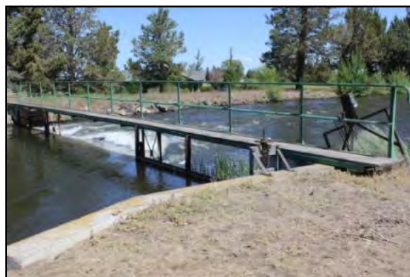
Catwalk, weirs, and headgate to Bear Creek Ranch ditch, looking northeast. 68
