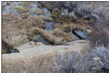
The headgates at Stearns Waste can discharge water from the canal to COID scrub land in an emergency. 68
