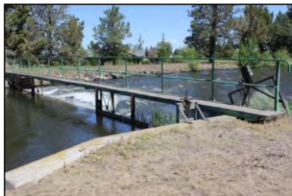
Catwalk, weirs, and headgate to Bear Creek Ranch ditch, looking northeast. 69
