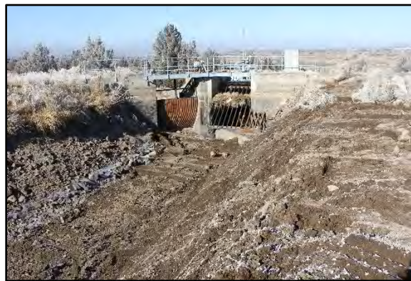
The intake structure with a trash rack to keep debris out of the steel pipe that crosses the Dry River bed. The wastewater spillway gate is on left. Photo shows recent major alterations to the canal bed and side slope. 408
