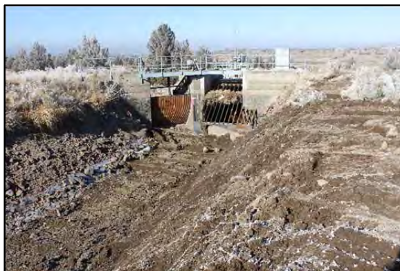
The intake structure with a trash rack to keep debris out of the steel pipe that crosses the Dry River bed. The wastewater spillway gate is on left. Photo shows 2017 major alterations to the canal bed and side slope. 3
