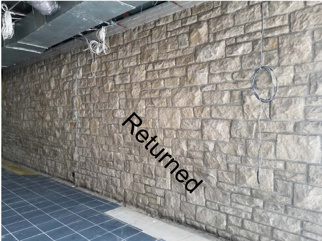
Figure 18. Lee's Summit Post Office. East wall of lobby after exploratory demolition of 1998 retail area, July 2017. Rosin Preservation.
