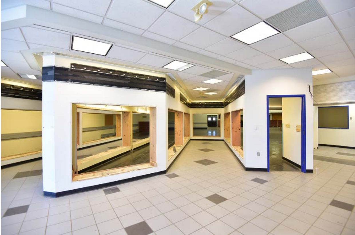
Figure 19. Lee's Summit Post Office. Lobby, post office box walls, view southwest. F-stop Photography, 2017.
