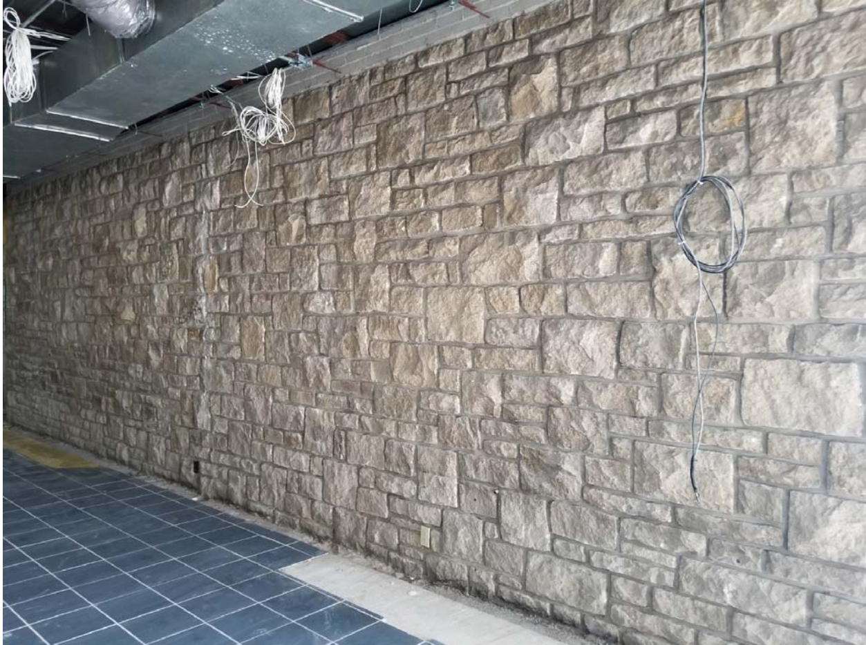
Figure 18. Lee's Summit Post Office. East wall of lobby after exploratory demolition of 1998 retail area, July 2017. Rosin Preservation.
