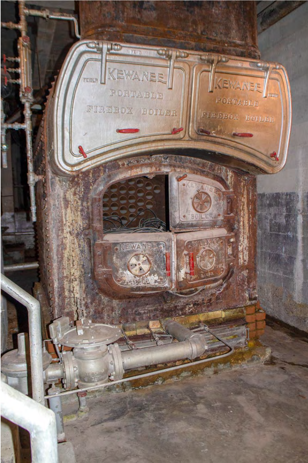
Photo 14: Boiler, view in basement. Camera facing east.
