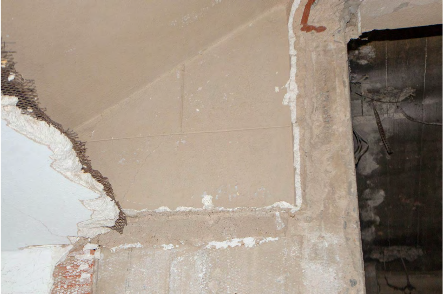
Photo 18: Detail view of Caen stone plaster treatment fragment. Camera facing west at stair.
