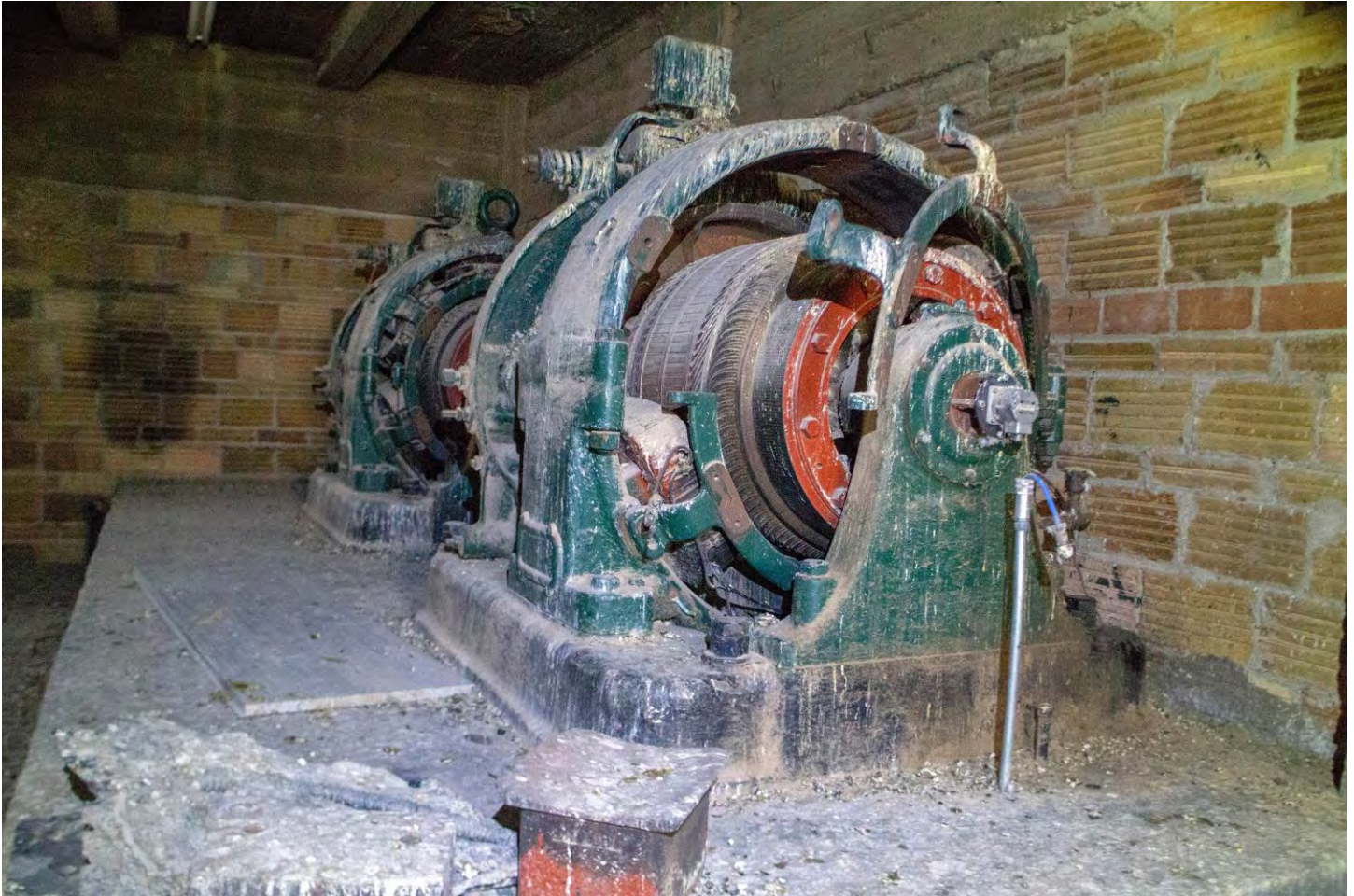
Photo 28: Elevator equipment in penthouse. Camera facing southeast.
