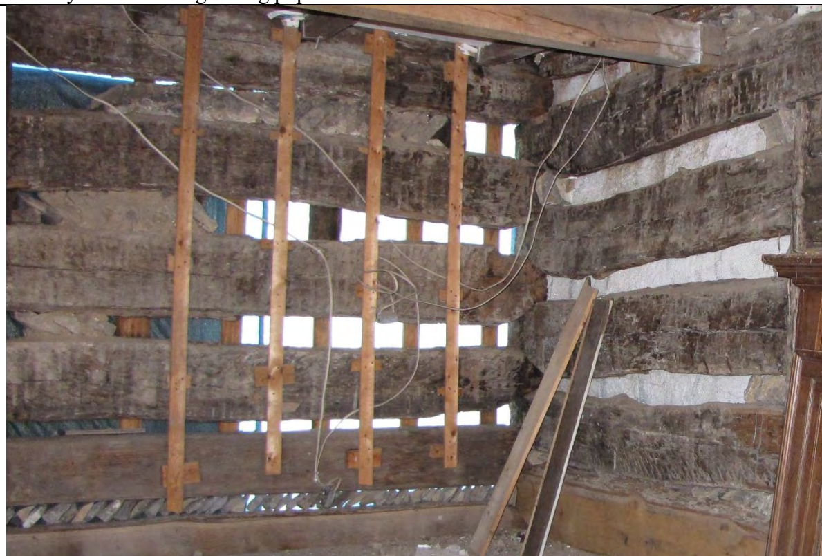
Interior corner of Willis Russell Memorial House. Note the large and irregular shaped gaps between logs.
