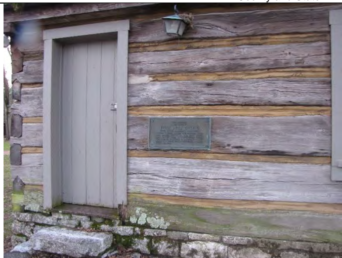
Restored original Post Office from Constitution Square, with uniform gaps between logs.
