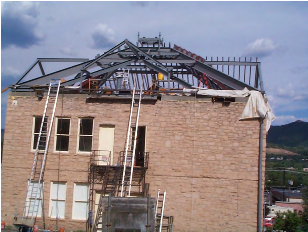
HP8. 8. The Animas City School/ Animas Museum in 2006 during the reconstruction of the hip-style roof. Camera looking east
