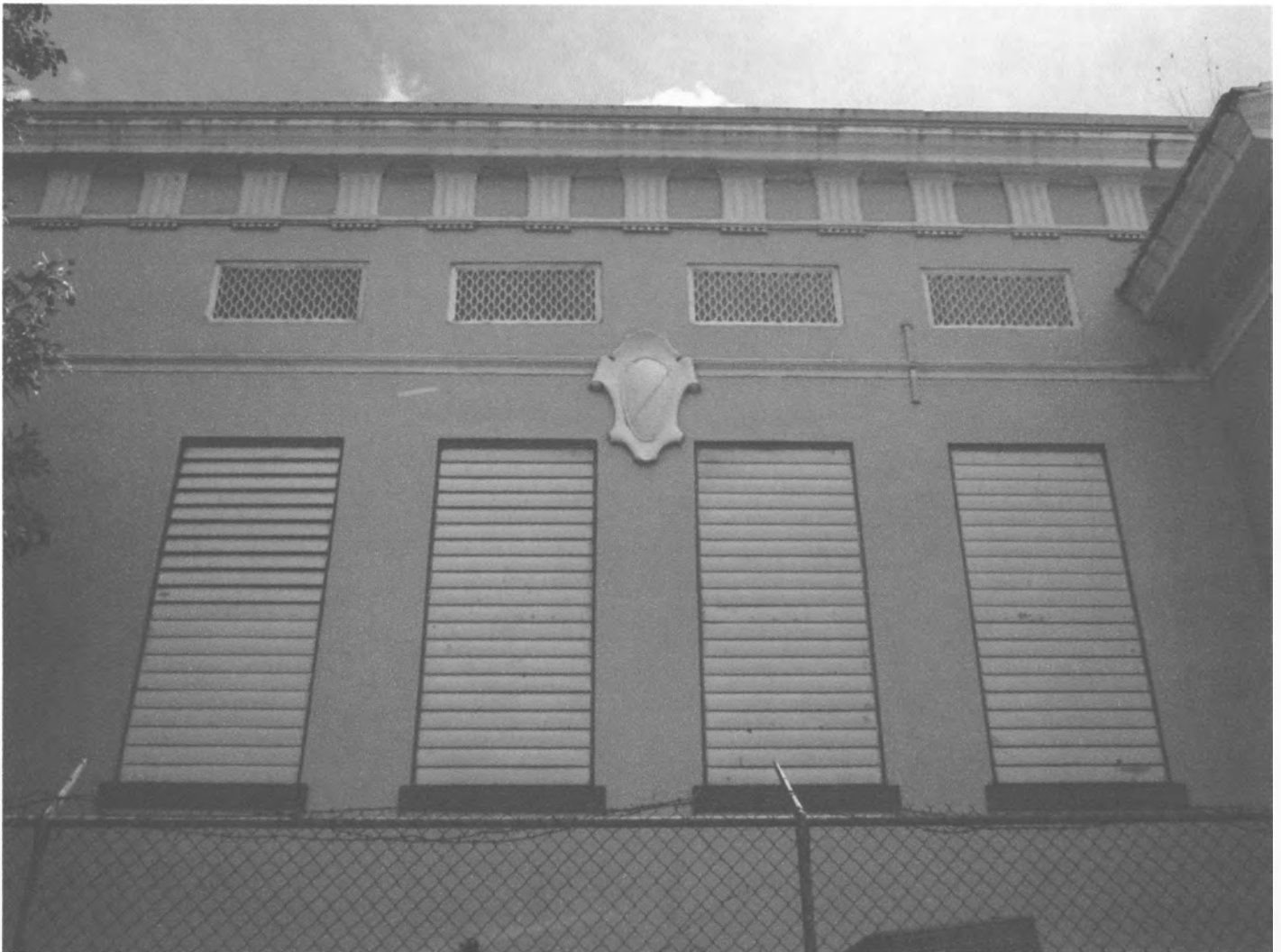
FIG. 6: Luis Muñoz Rivera School west elevation, looking northeast - portico detail, in Lajas Puerto Rico. Four equally spaced, rectangular, vertical window openings are located at either side of the portico. A cartouche above each set establishes local symmetry at these sections of the façade. A lean molding strings together triglyphs and metopes and below a line of terracota ventilators. Photo: Eduardo Miranda, October 24, 2012. Source: Jorge Rigau Arquitectos, San Juan Puerto Rico.
