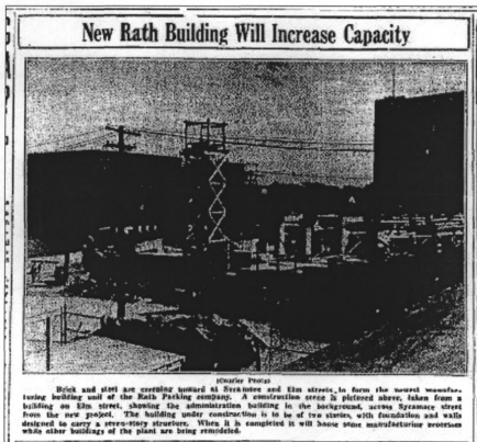
Figure 15: New warehouses going up to the southwest of the Administration Building (rear left) ( Waterloo Daily Courier , August 11, 1937)
