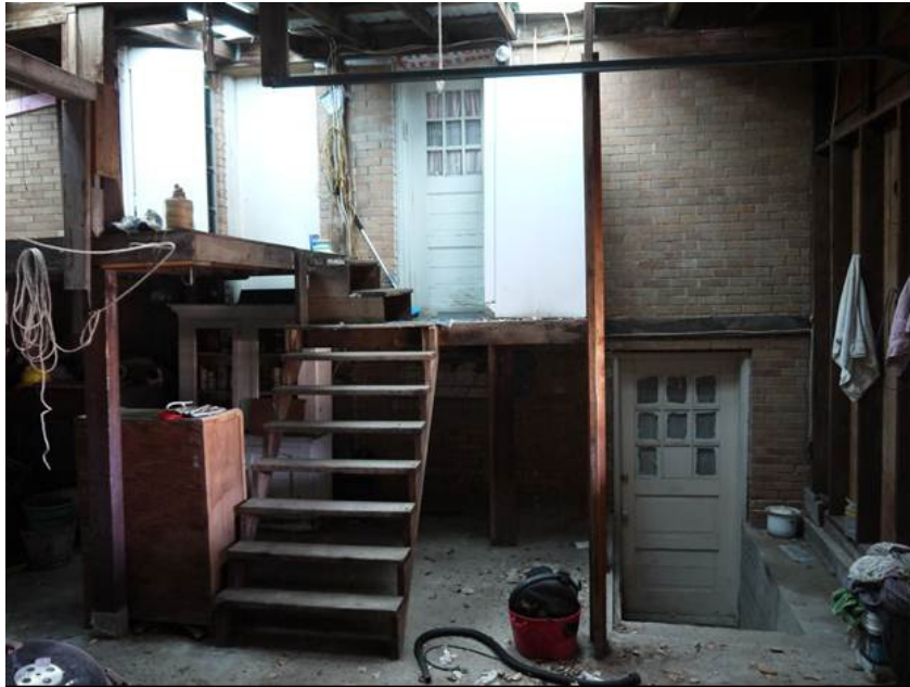
Photo #0006: West elevation, detail of doors in west elevation of school building. View to the east.
