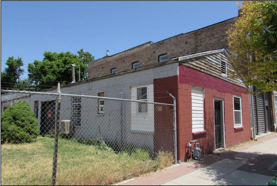
Photograph 21 of 34: Post-WWII style Service Bay/Business; 568 W. 200 S., south (right) and west elevations; camera facing northeast
